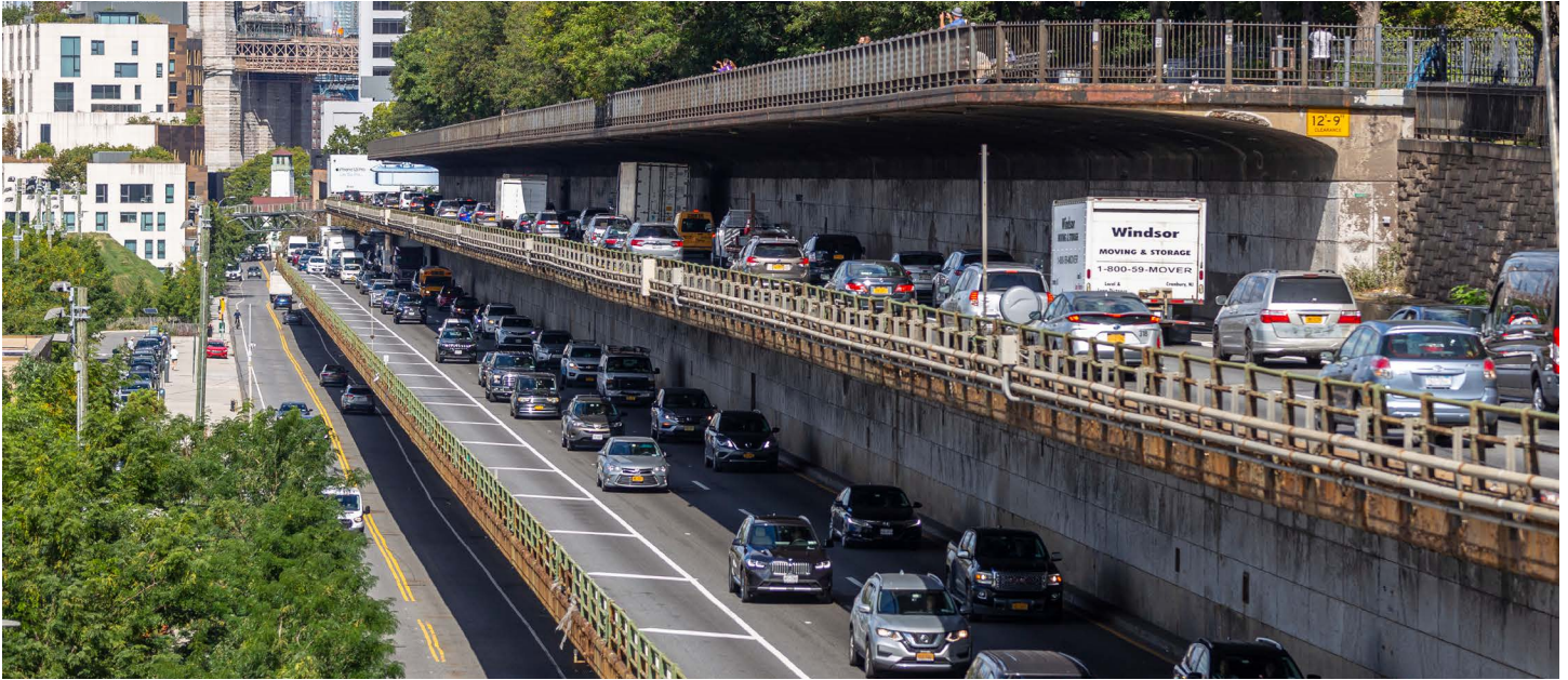
The Triple Cantilever of the Brooklyn-Queens Expressway (BQE), which is due for extensive upgrades and repairs.
