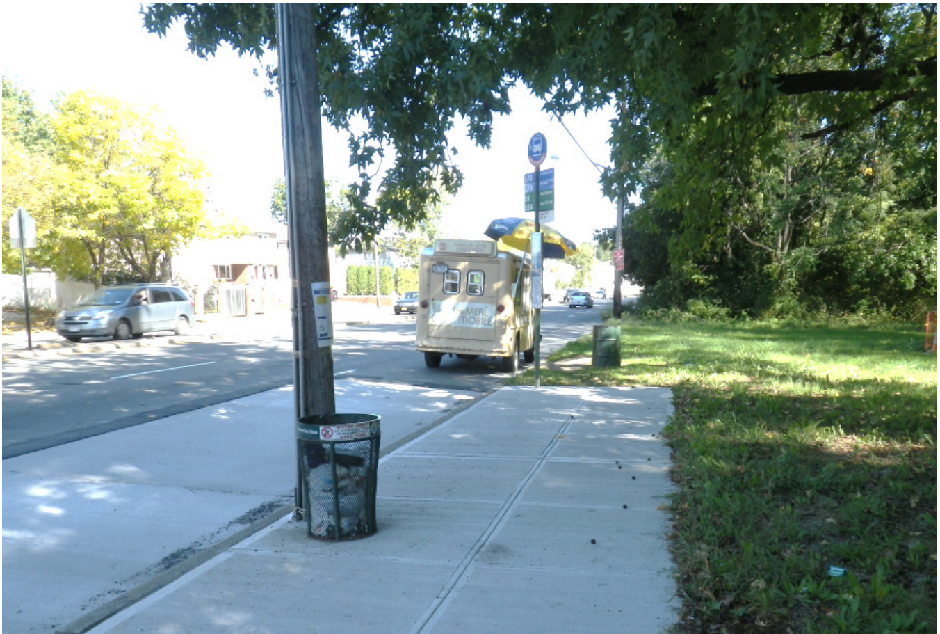
Figure 4 – New sidewalk constructed for bus stop previously in dirt path, new concrete bus pad
