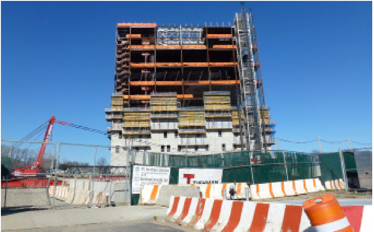
FIGURE 5 | The Public Safety Answering Center II (PSAC II), currently under construction. When it opens its doors in 2015, it will house approximately 850 employees.
