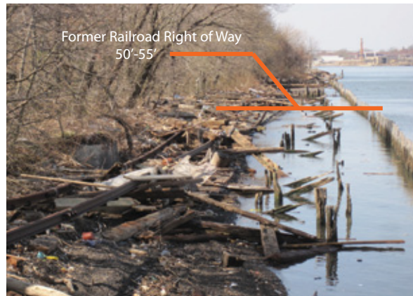
Railroad right-of-way above eroded shoreline
