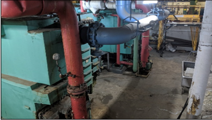
Photograph 5. Chiller equipment, domestic water and steam piping in the Property building basement.
