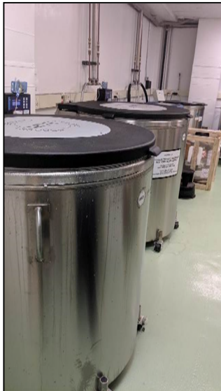
Photograph 7. Research freezer/refrigeration units in the basement
