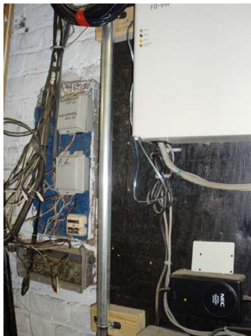
Photograph 34 – Electrical Equipment – Building No. 2
