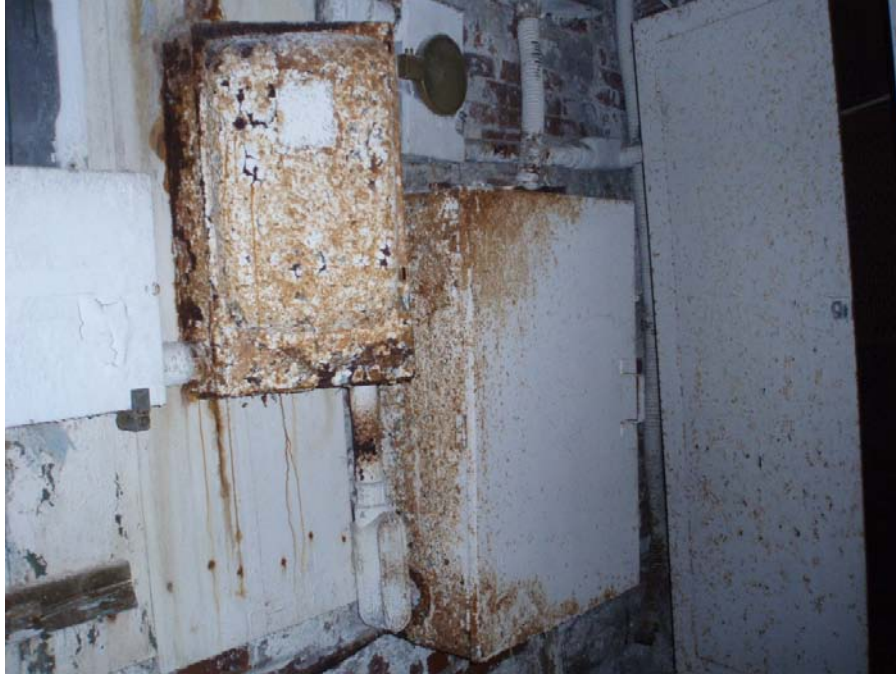
Photograph 17 – Electrical Equipment – Building No. 1
