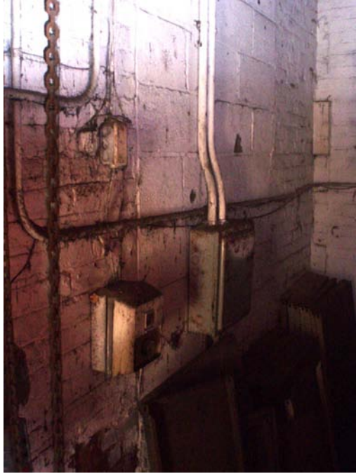
Photograph 11 – Electrical Equipment - Building No. 1
