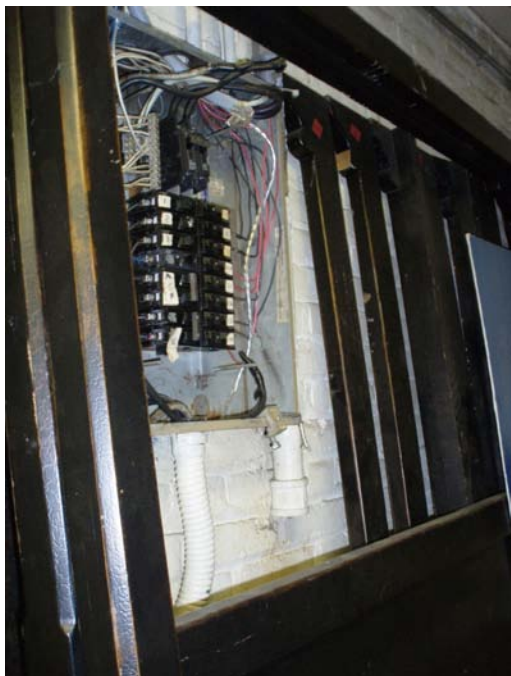
Photograph 35 – Electrical Equipment – Building No. 2
