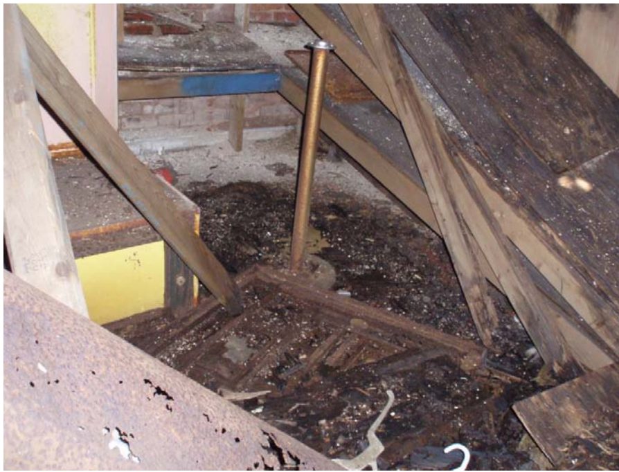
Photograph 12 – Miscellaneous Trash - Building No. 1
