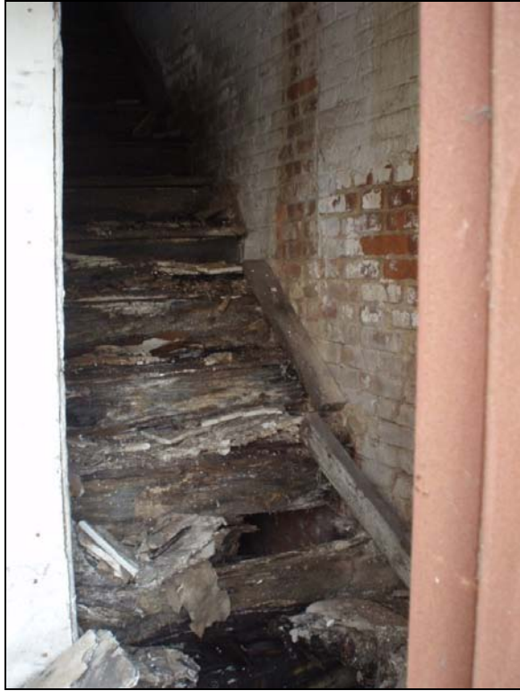
Photograph 3 – Dilapidated Staircase - Building No. 1
