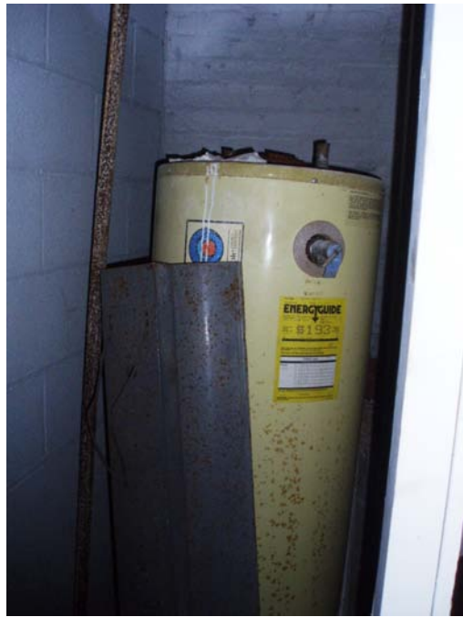
Photograph 14 – Hot Water Heater - Building No. 1
