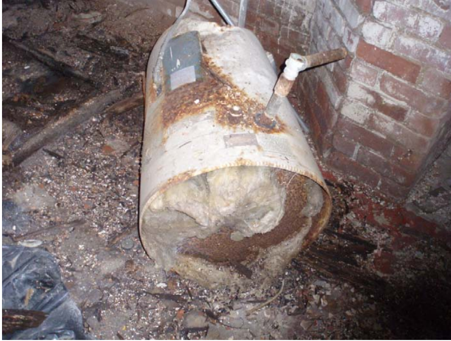
Photograph 5 – Hot Water Heater - Building No. 1
