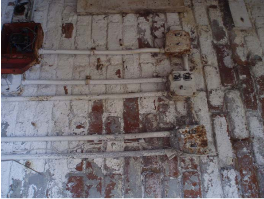
Photograph 23 – Electrical Equipment – Building No. 1
