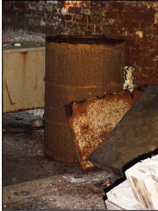
Photograph 25 – Rusted Drum – Building No. 1
