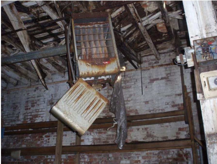
Photograph 6 – Electric Heater - Building No. 1
