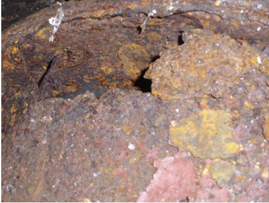
Photograph 15 – Rusted Drum – Building No. 1
