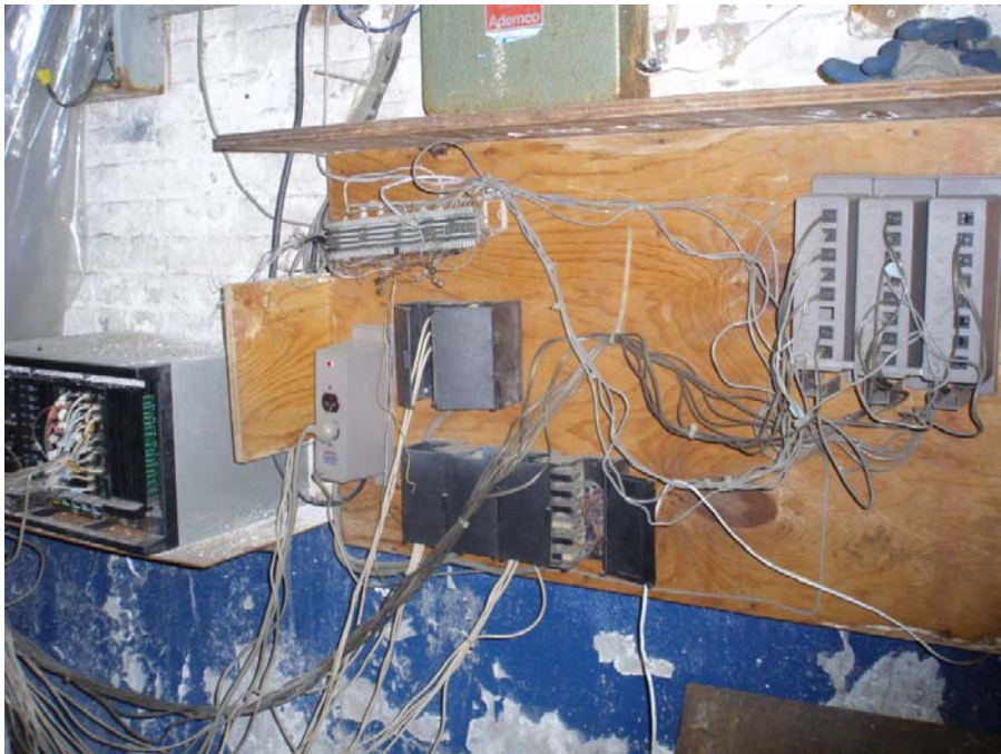
Photograph 36 – Electrical Equipment – Building No. 2
