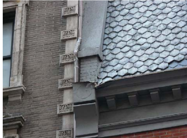
Sheet metal damage and missing slate tiles at Mansard roof
