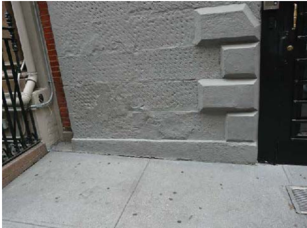
Stone deterioration is visible through paint
