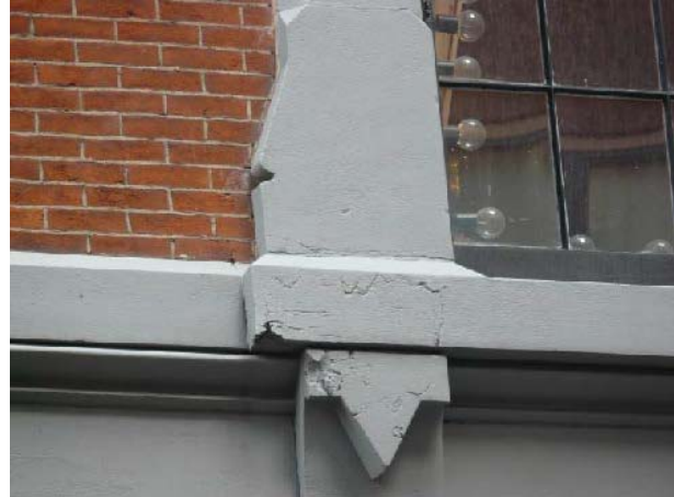
Stone damage is present and visible
