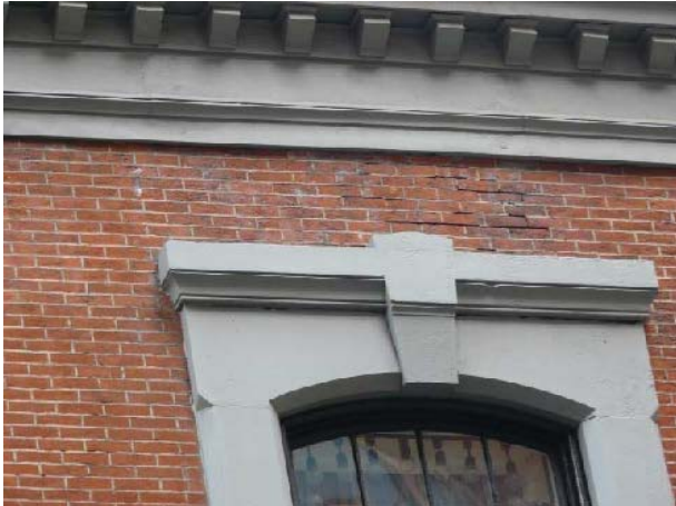
Brick soiling and efflorescence through open mortar joints
