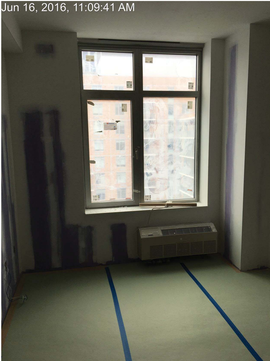
Interior of Apartment 14P showing PTAC and Apartment Window
