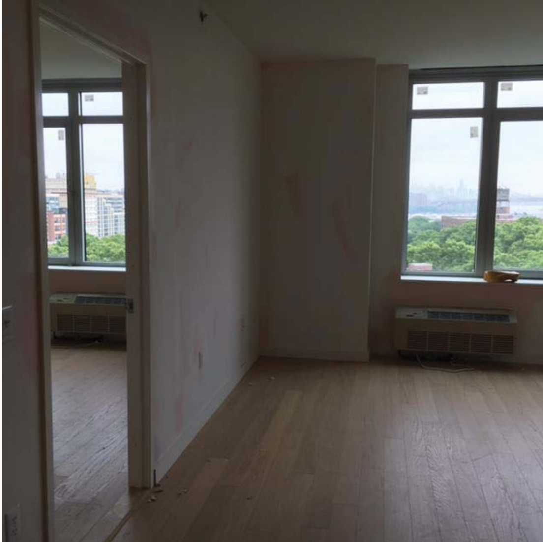
Interior of Apartment 11C showing PTACs and Apartment Windows
