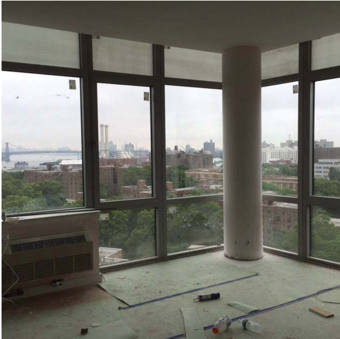
Interior of Apartment 14F showing PTAC and Apartment Windows
