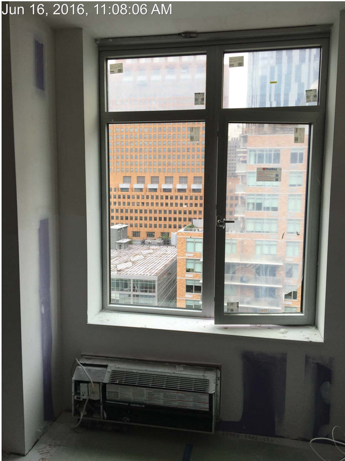
Interior of Apartment 15P showing PTAC and Apartment Window
