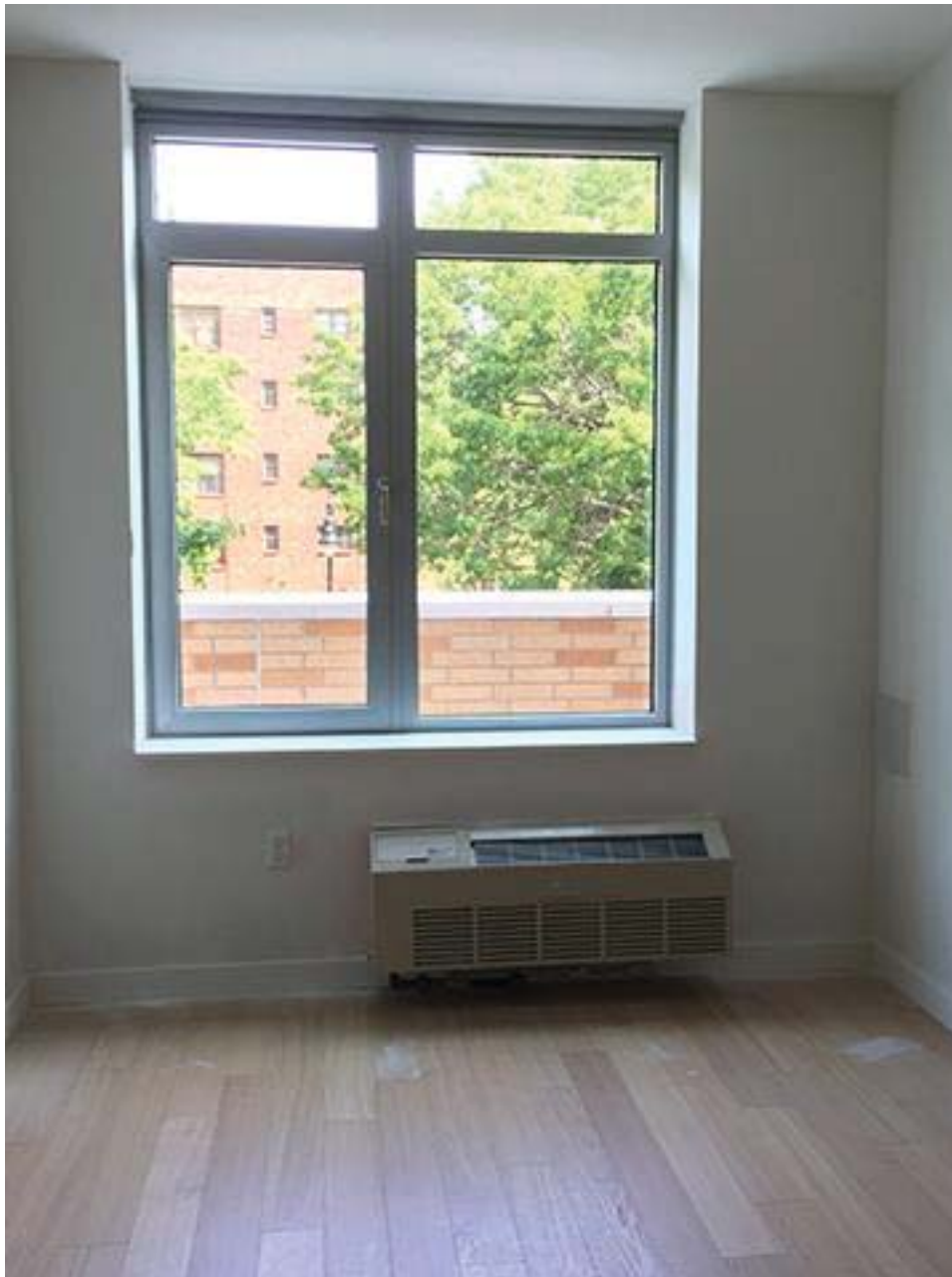
Interior of Apartment 2C showing PTAC and apartment window
