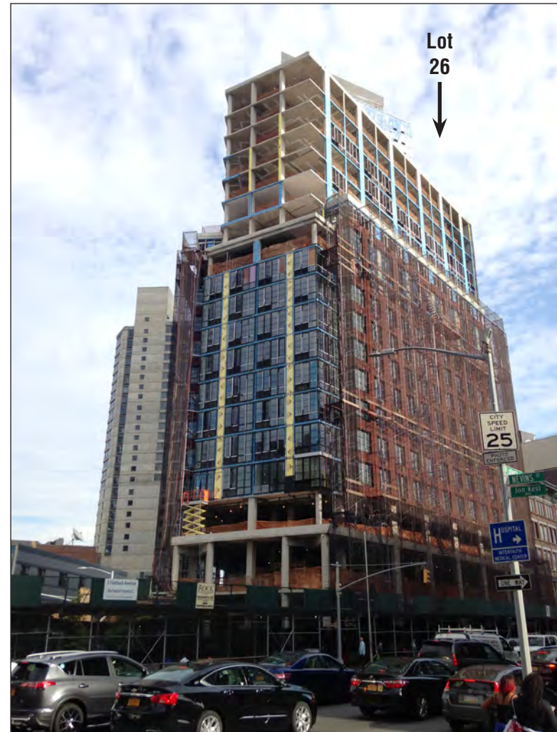
Lot 26 in the Project Area is under construction with a 19-story building. View from Fulton Street and Nevins Street facing southeast. 2
