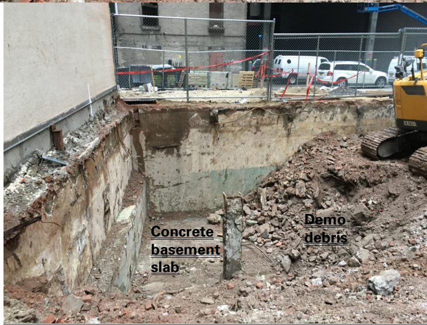
Photograph 2 – View of sloped excavation for TP-1 and TP-2, facing northeast. The sloped excavation occurred entirely above the existing cellar slab; therefore above any potentially sensitive archaeological zone. The material above the slab was demolition debris. The concrete slab is shown in the base of the sloped excavation. Photo taken 12/7/2016.
