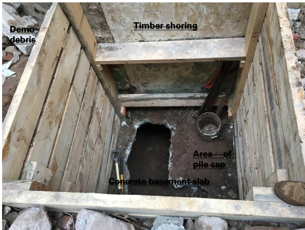
Photograph 1 – Overhead view of Feb 2016 geotechnical test pit excavation. The timber shoring boards extend from current grade to the top of the concrete basement slab (12 feet below grade). After breaking through the concrete slab, hand excavation continued to 23 feet below grade through grayish-brown clayey silt. No cultural material or historical structural elements were reported during this hand excavation. Photo taken 2/19/2016.
