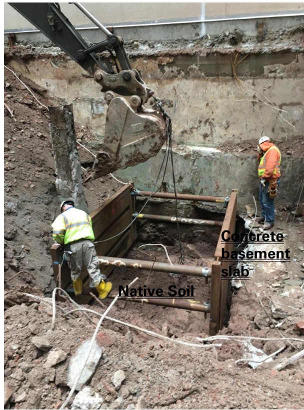
Photograph 3 – View of TP-2 facing north, showing excavation through and below the concrete slab into the potentially sensitive archaeological zone, Sheet piling allowed for a much more limited excavation at the archaeologically sensitive depth. No cultural material or historical structural elements were reported below the existing basement slab. Photograph taken 12/7/2016.
