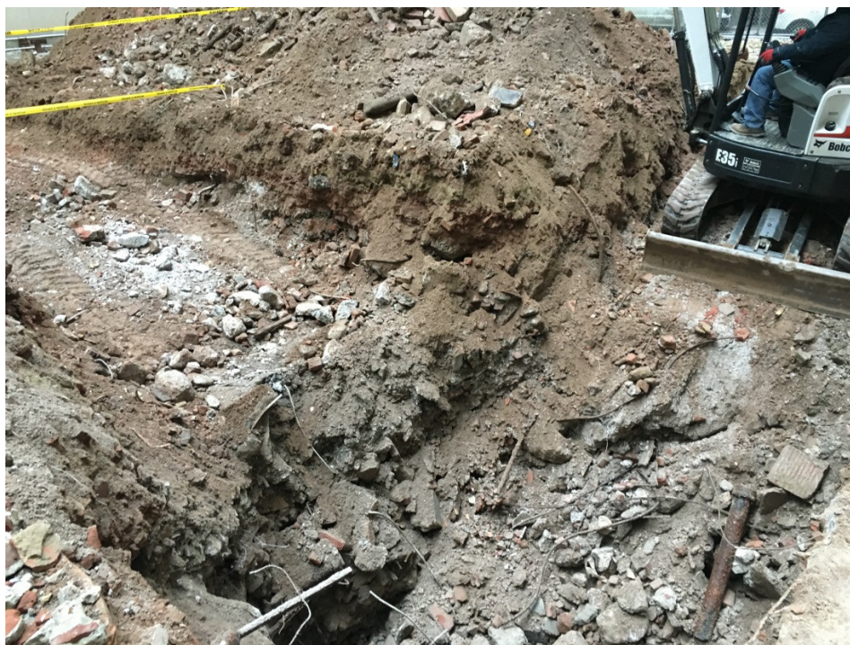
Photo 002: General view of the demolition debris excavated from the test pit, facing northeast.
