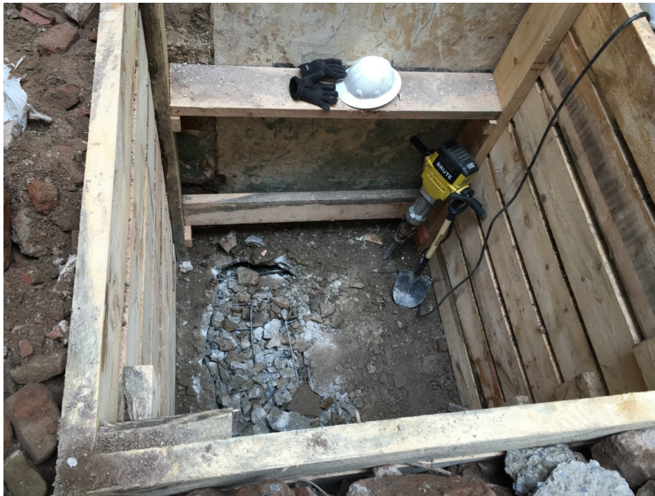
Photo 004: General view of the test pit showing rebar found underneath the 9-inch-thick concrete slab, facing southwest.
