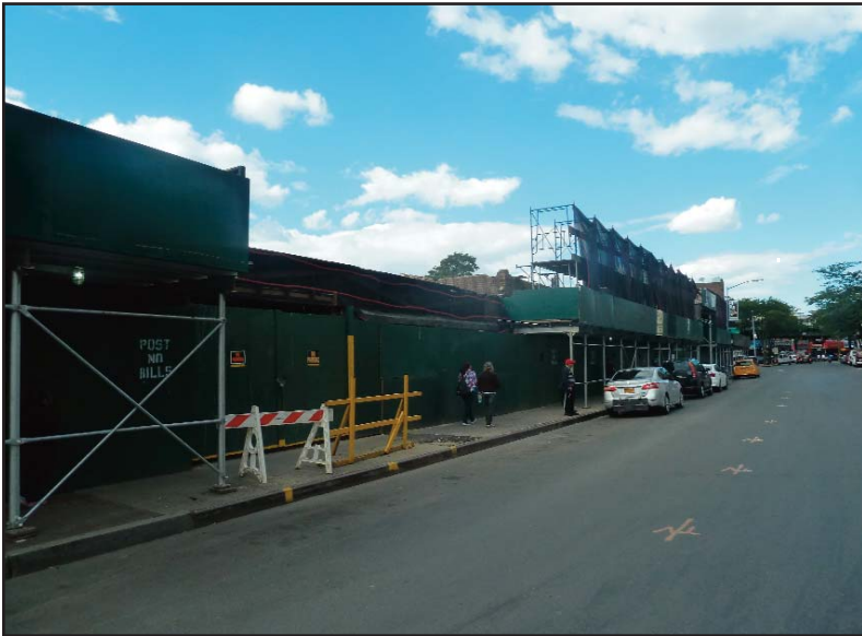
3. View from Baxter Avenue (just north of Ithaca Street) looking northwest towards proposed development site.
