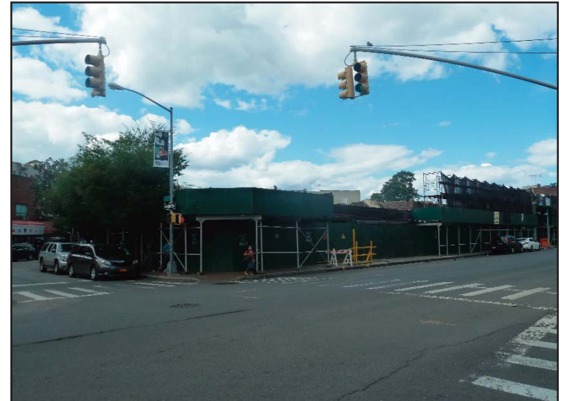
4. View from corner of Ithaca Street and Baxter Avenue looking northwest towards proposed development site.
