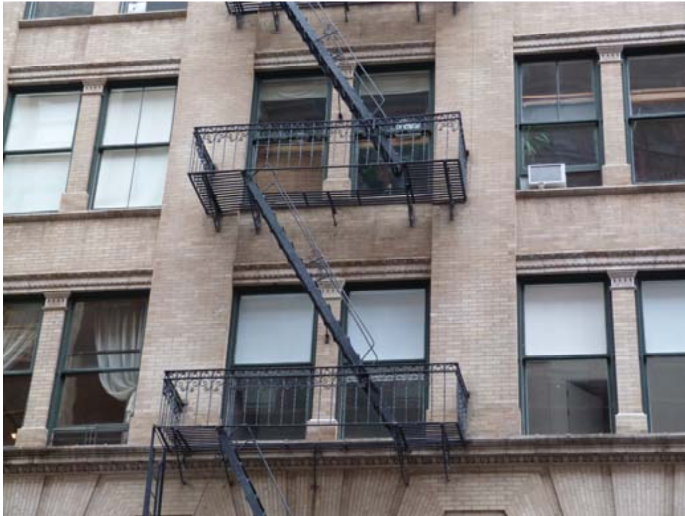
Deteriorated Wood Windows and Restored Fire Escape on Bleeker Street
