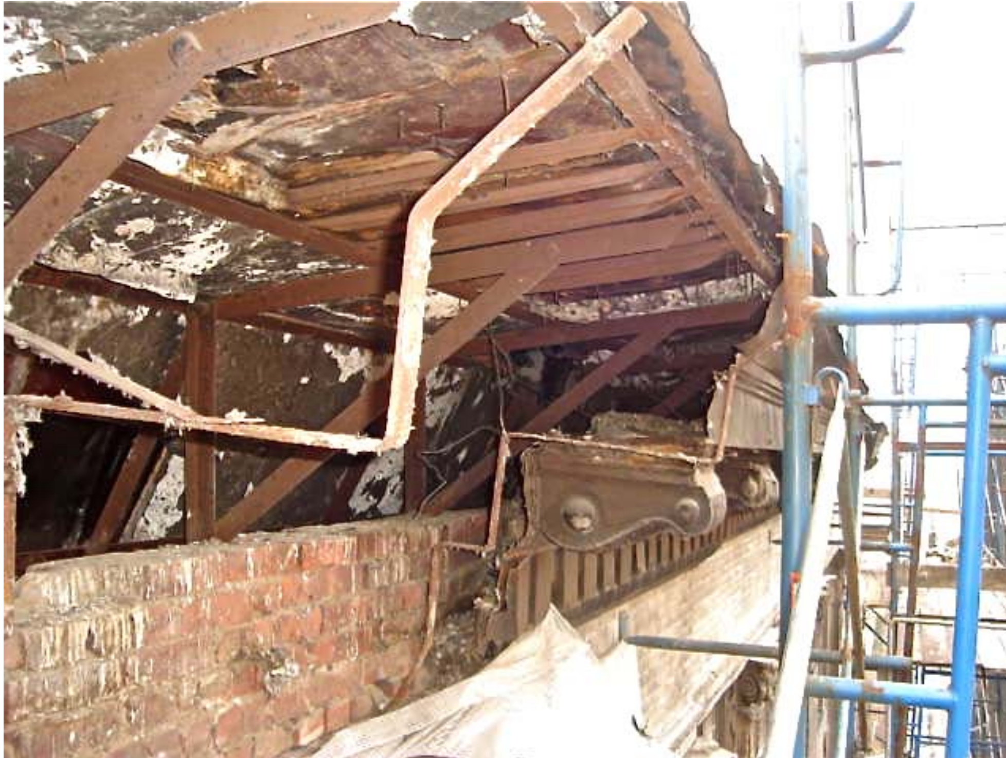
Original cornice assembly condition exposed during cornice replacement work performed on April 2006
