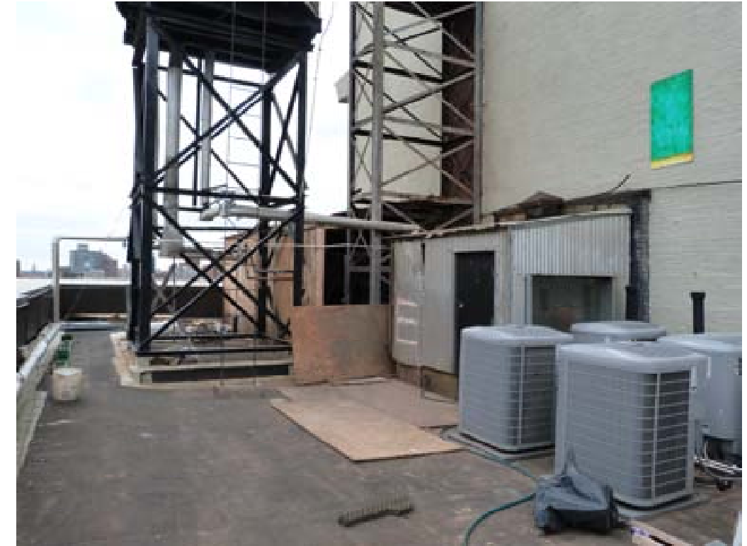
Bulkheads, Mech. Equipment, and Water Tank at East end of roof
