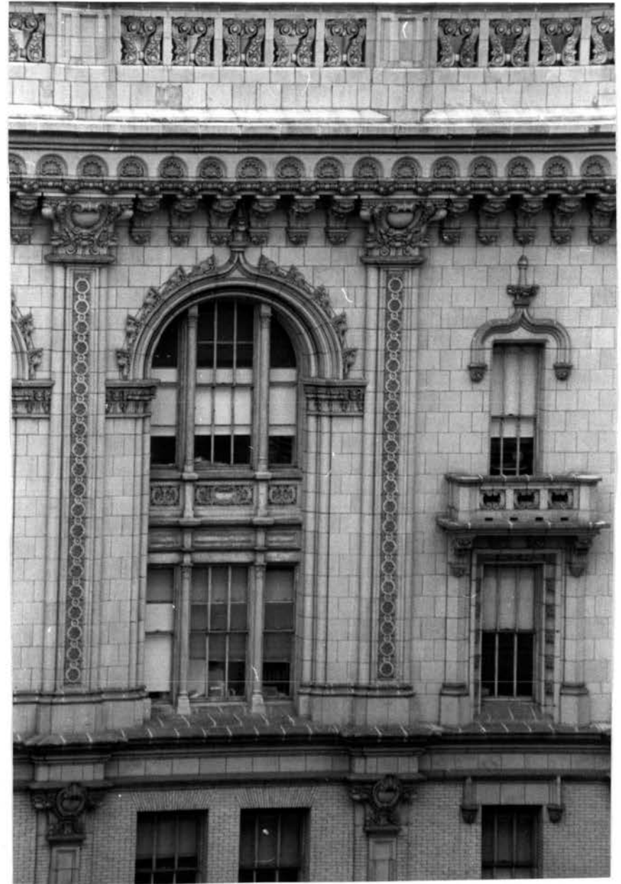
New York Times Building (originally Times Annex) 43 rd Street facade, detail Photo: Carl Forster
