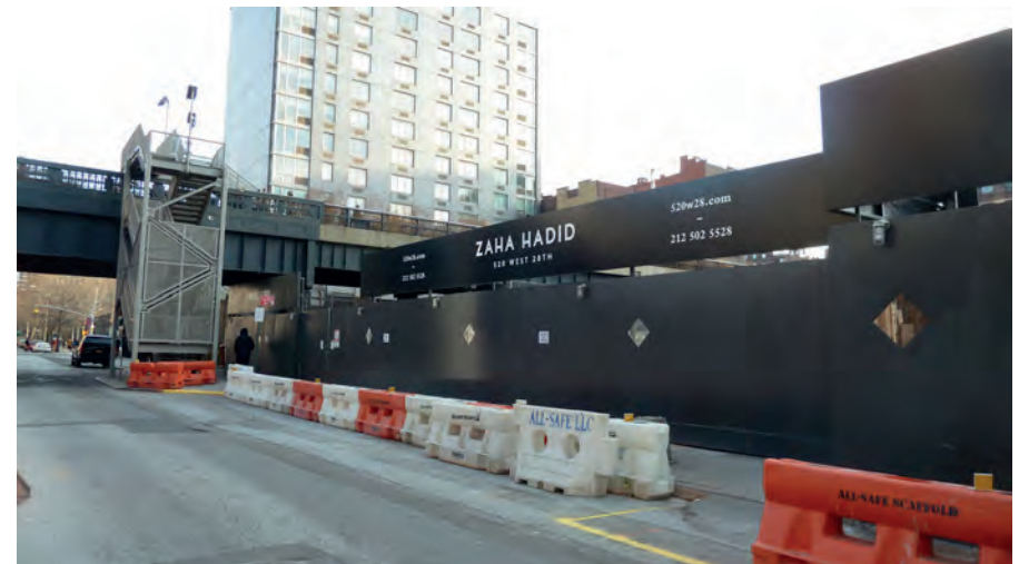
4. View of construction at Development Site looking south/southeast from W 28th Street
