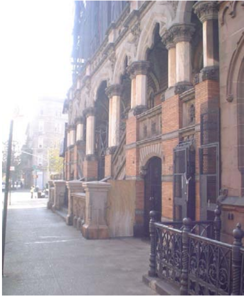
Sidewalk conditions in front of former St.Thomas Church
