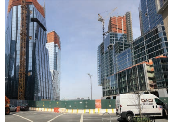
Riverside Center, a multi-building Large-scale General Development, under construction on the Upper West Side of Manhattan
