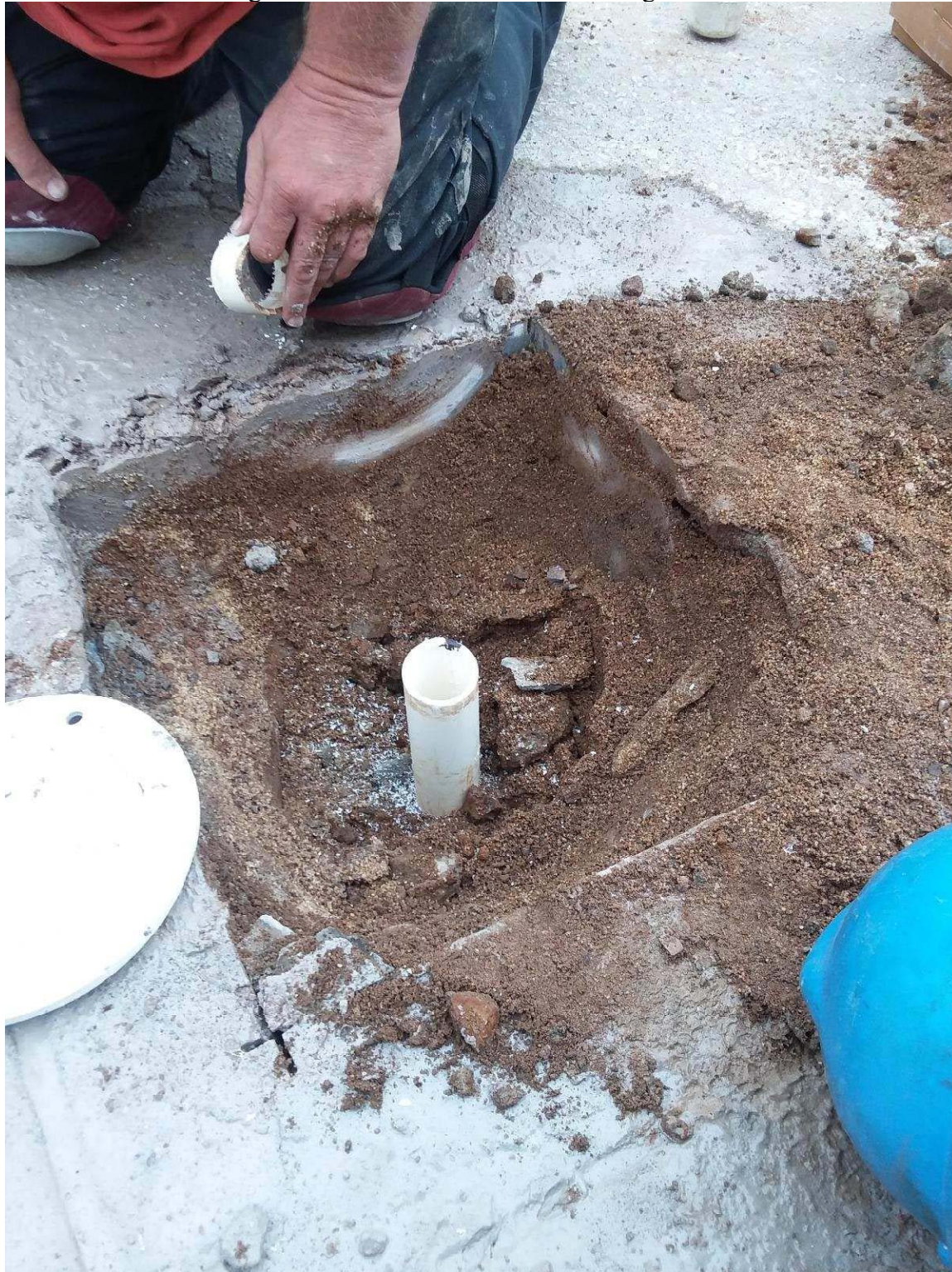
Photo 1: MW-02 damaged manhole removed and well casing cut down
