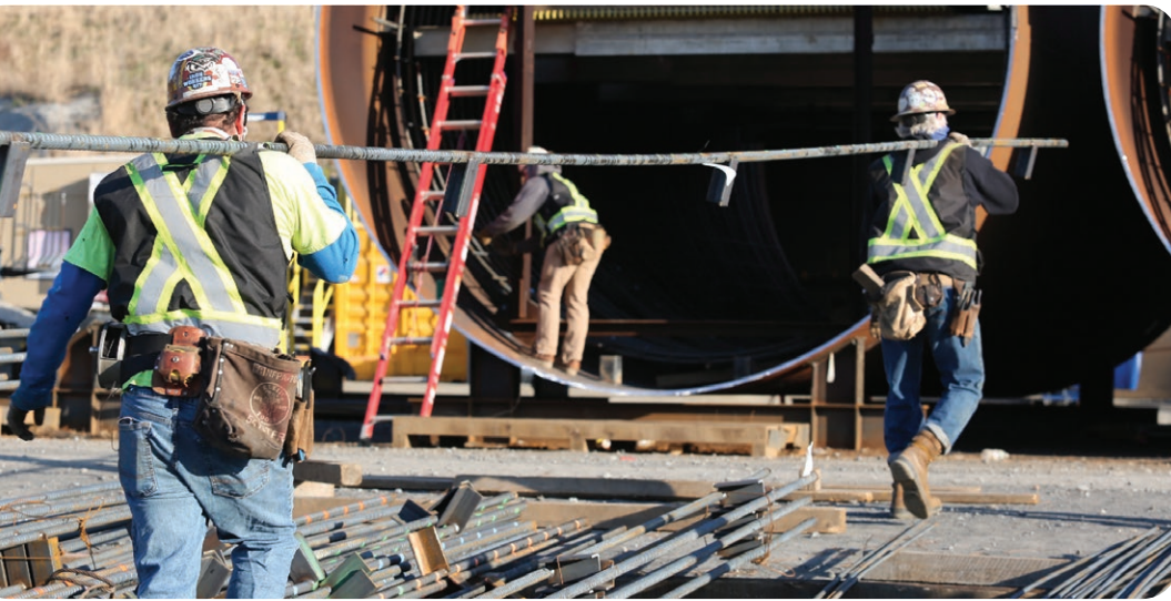
Work on steel liners for the Delaware Aqueduct Bypass Tunnel (each liner section is 16' in diameter and 40' long)
