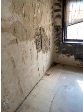
Abated plaster wall (Building 2, Apt. 3A)
