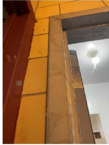
Abated door frame (Building 2, Apt. 3A)
