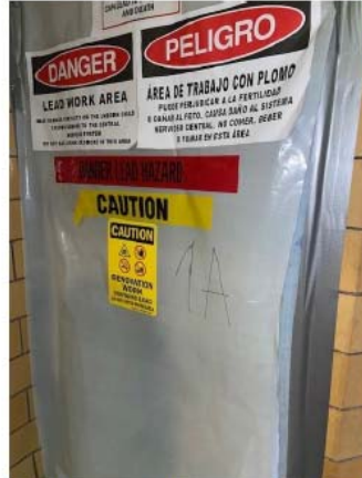
Entrance Critical Barrier (Building 3, Apt. 1A)
