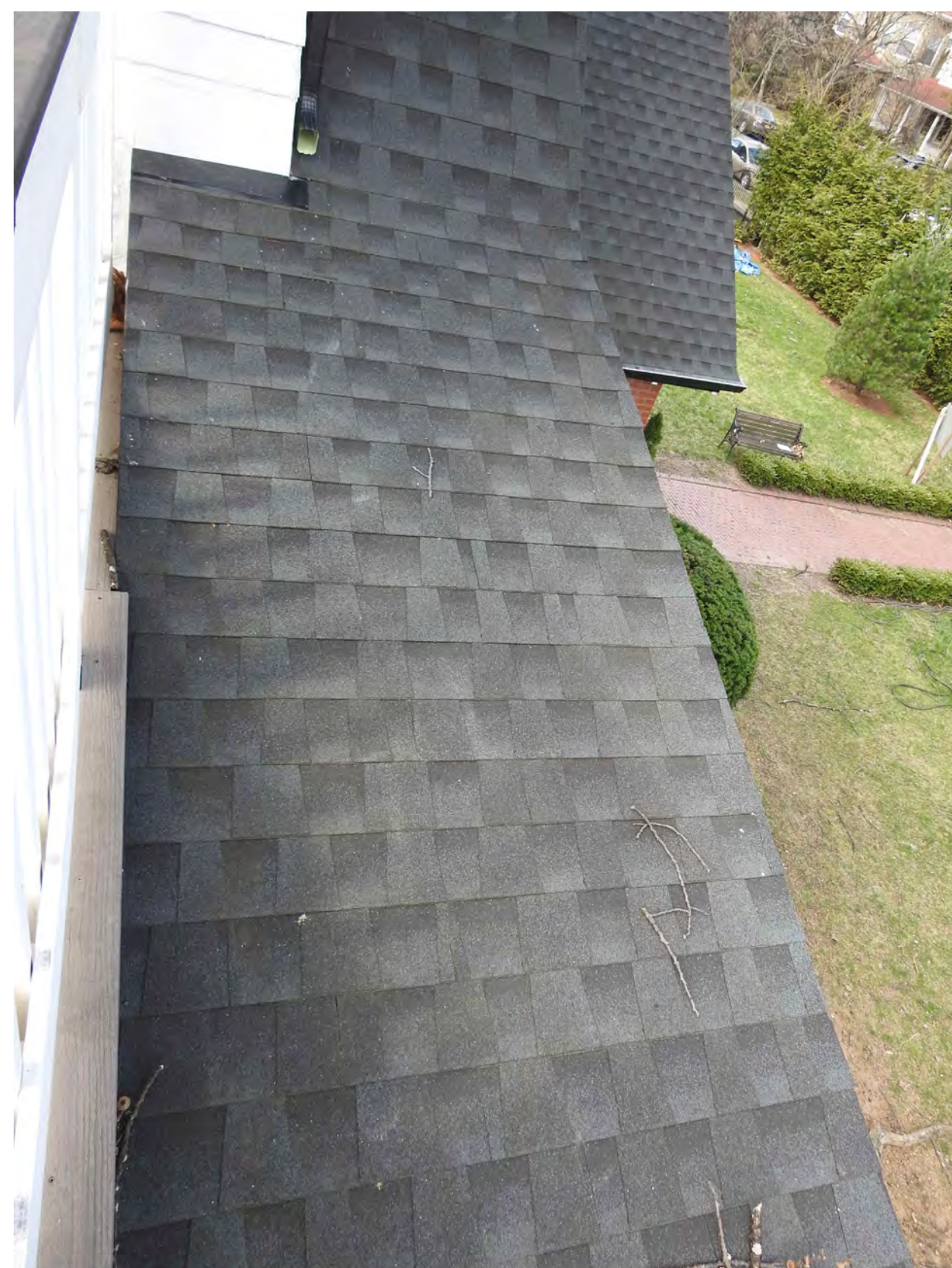
EAST FACADE - VIEW OF ROOF LINE OVER DECK/RAILINGS FACING THE NORTH/FRONT FACADE
