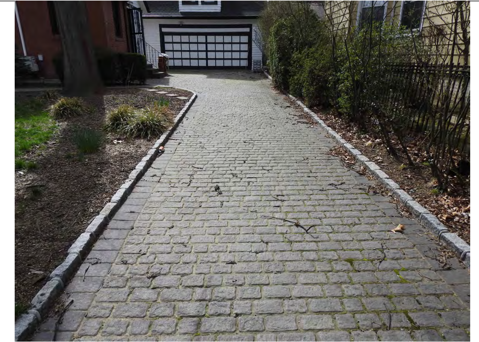
DRIVEWAY PAVEMENT CHANGED IN 2020 (PHOTO FROM GOOGLE VIEW IN 2020)
