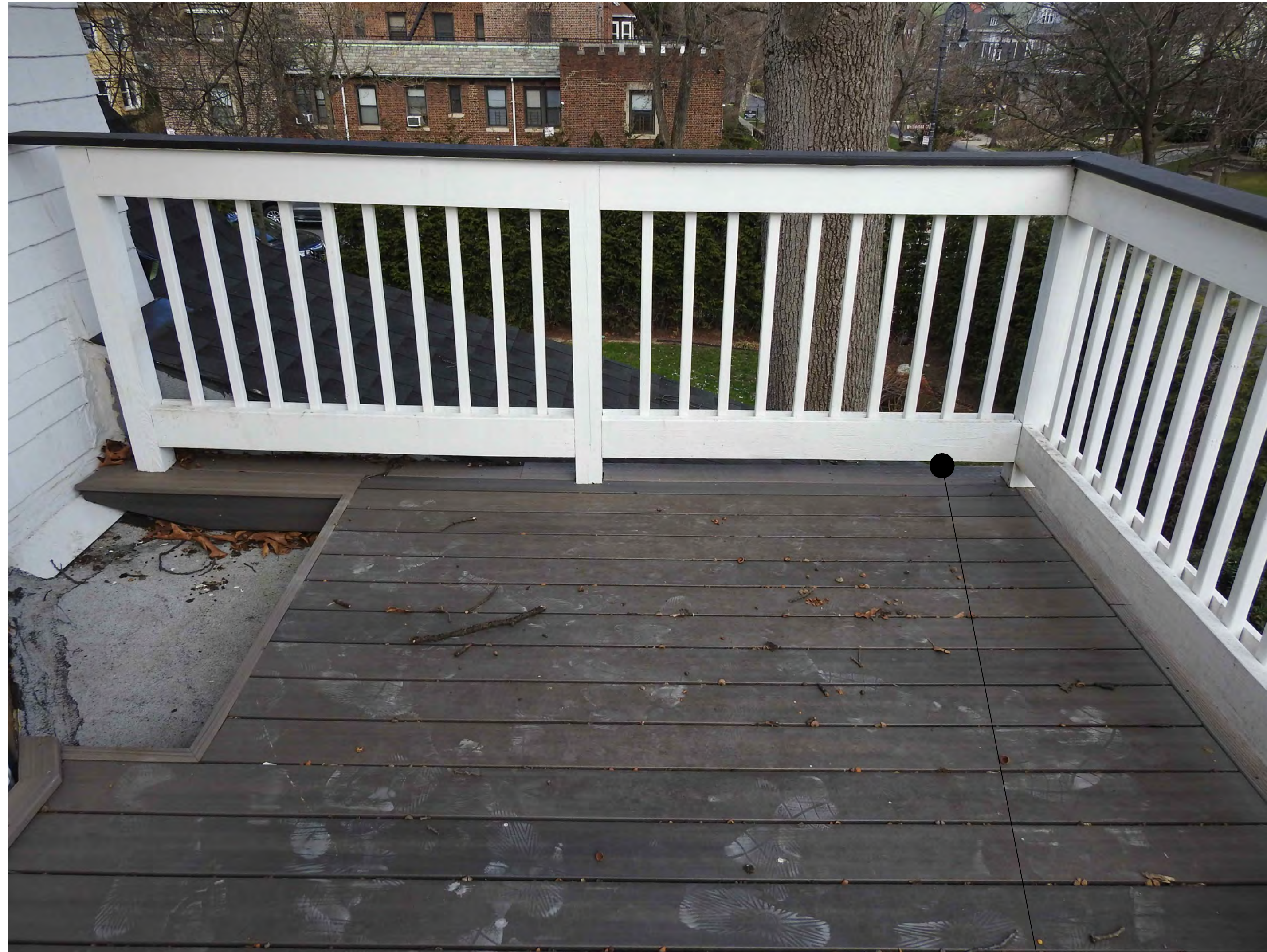
EAST FACADE - VIEW FROM EXISTING ILLEGAL WOOD DECK & BALCONY RAILINGS TO INTERIOR (PHOTO FACING EAST & FRONT/NORTH FACADE)
