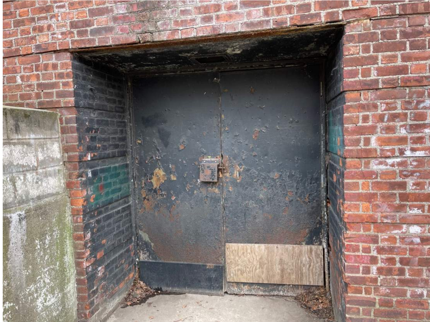
EXISTING DOUBLE DOORS AT THE FILTER BUILDING
