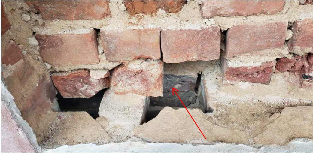
Exterior View: showing cavity in the wall
