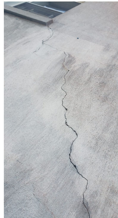
230 exterior View: showing cracks
