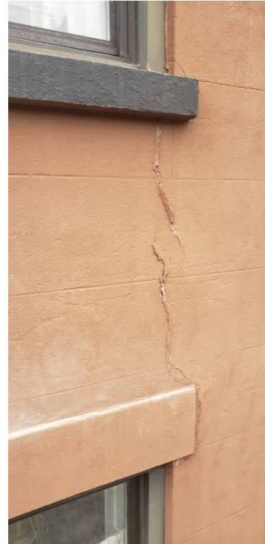
Exterior View: where vertical cracking has been observed Between the Third and Second Flrs,
