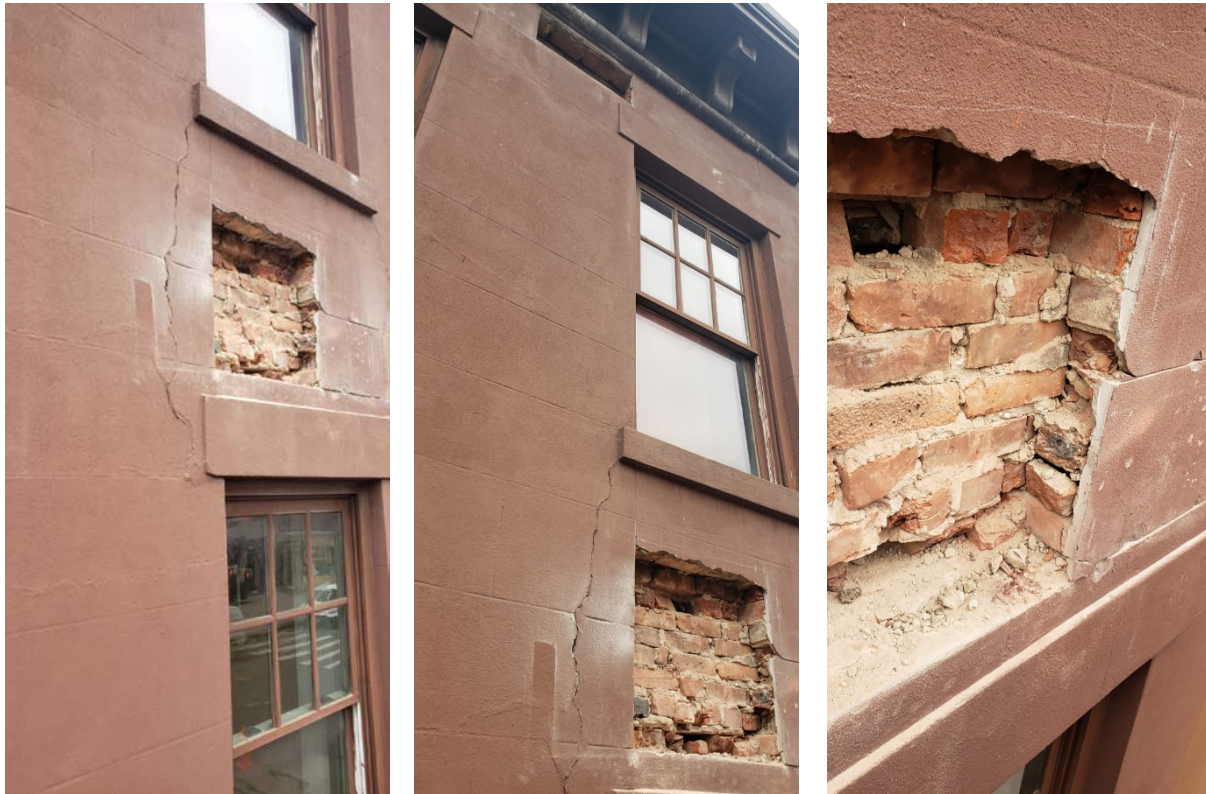
Exterior View: showing proposed enlargement probe #2, and vertical cracking between the 2nd and the 3rd floors
