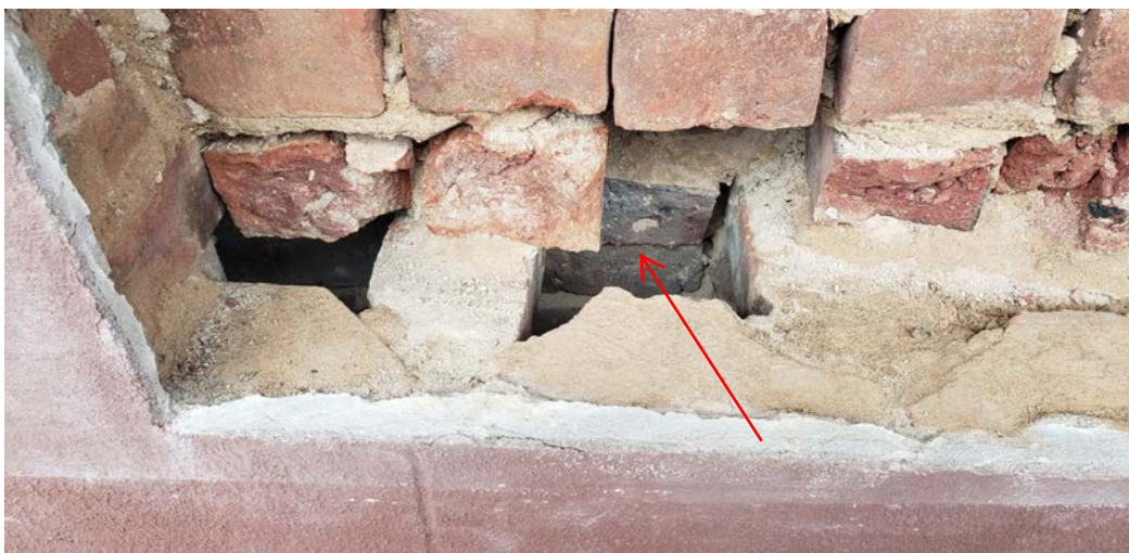
Exterior View: showing cavity in the wall
