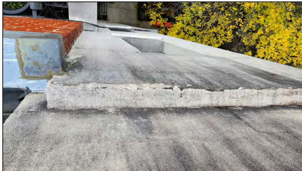
Ragged edges & discoloration of deteriorated EIFS
