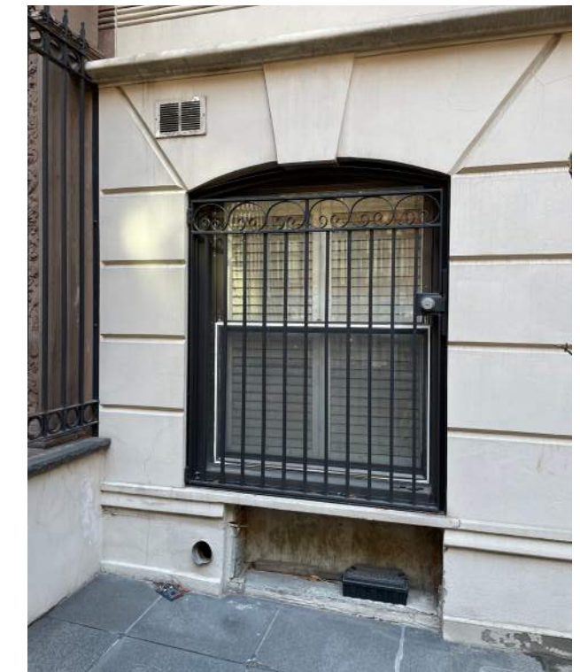
Missing Louver at 17 E77th Street
