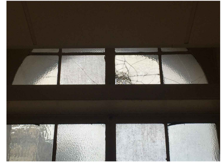
BROKEN AND CRACKED GLASS
