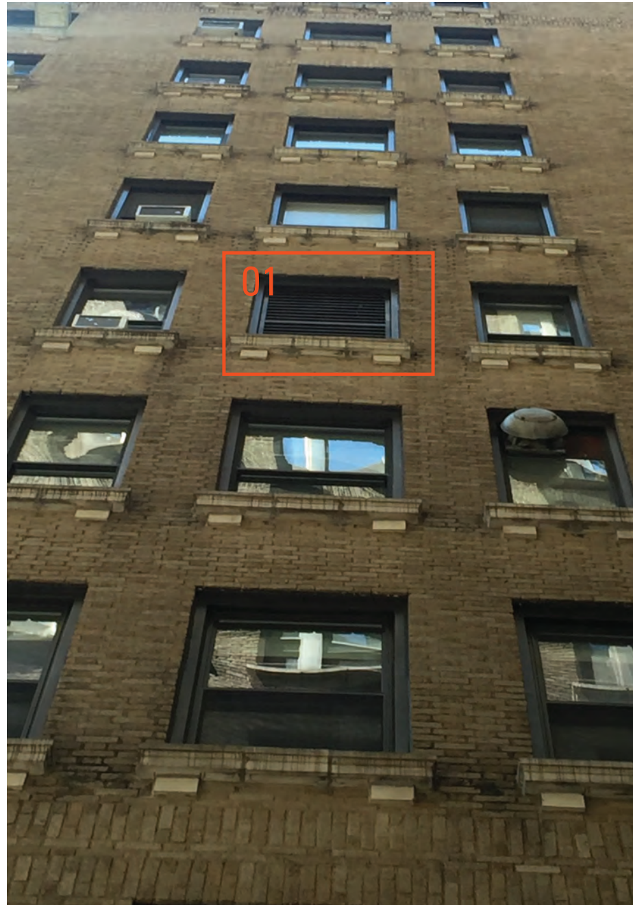
01 - (2) CONDENSING UNITS AT 6TH FLOOR WINDOW; FULL WINDOW
