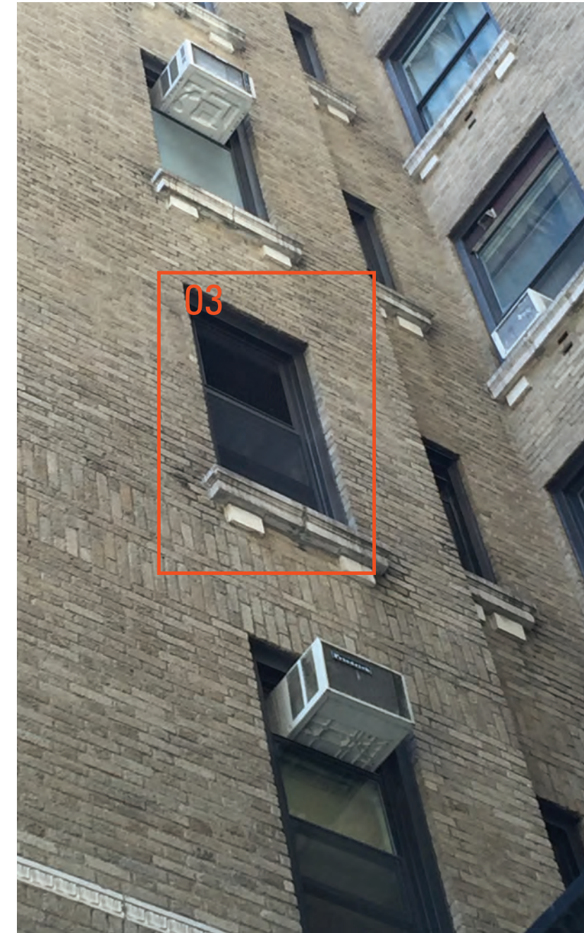
03 - CONDENSING UNITS AT 4TH FLOOR WINDOW; UPPER HALF WITH DOUBLE HUNG BELOW
