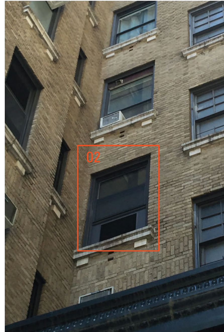
02 - CONDENSING UNIT AT 4TH FLOOR WINDOW; LOWER HALF WITH DOUBLE HUNG ABOVE
