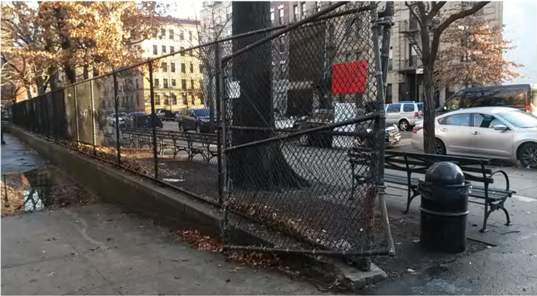
BROKEN 8FT CHAIN LINK GATE TO PLAYGROUND
