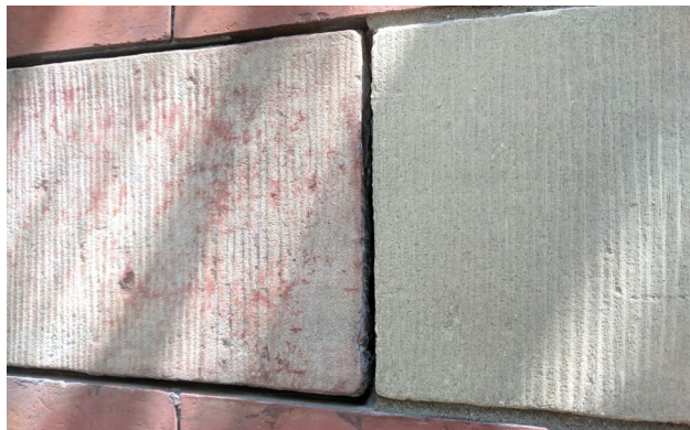
The color of the historic masonry on the left is matched by the mineral stain coating on the right.
