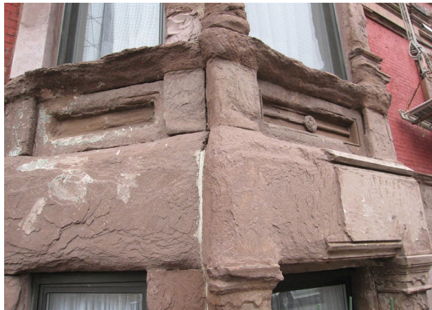
Significantly deteriorated brownstone, often referred to as delamination.
