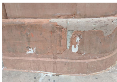
The patching material used here (the light colored areas) is not compatible with the original stone, was installed incorrectly, and was not tinted properly (the color is wearing off).
