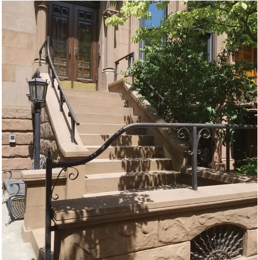
A simple metal railing has been installed on the top of this masonry stoop for safety.
