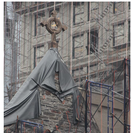
Fragile or deteriorated architectural features can be stabilized and protected in place, as seen here while construction is in progress.
