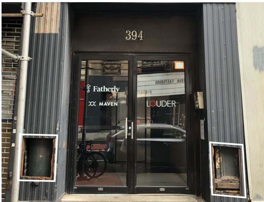
The historic storefront has been covered with metal cladding. Probes have revealed the original cast iron piers.
