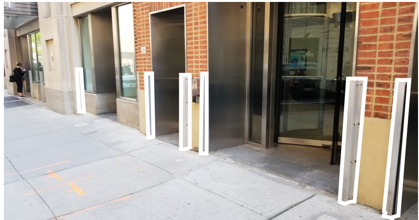
Posts for removable flood protection barriers, all with a neutral finish, installed at plain masonry at select openings.
