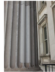
The light colored stone shown here is replacement stone installed as a Dutchman repair.
