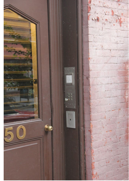
An intercom installed within a door opening.
