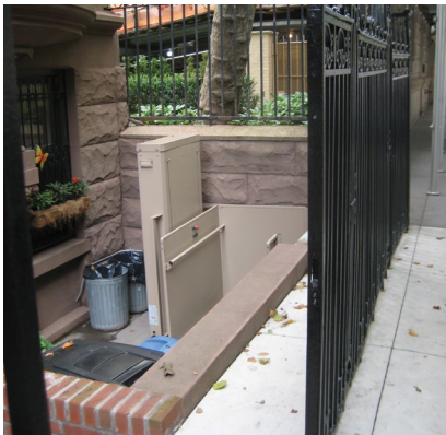
A metal platform lift installed within an areaway, finished to match the surrounding brownstone and screened by ironwork.
