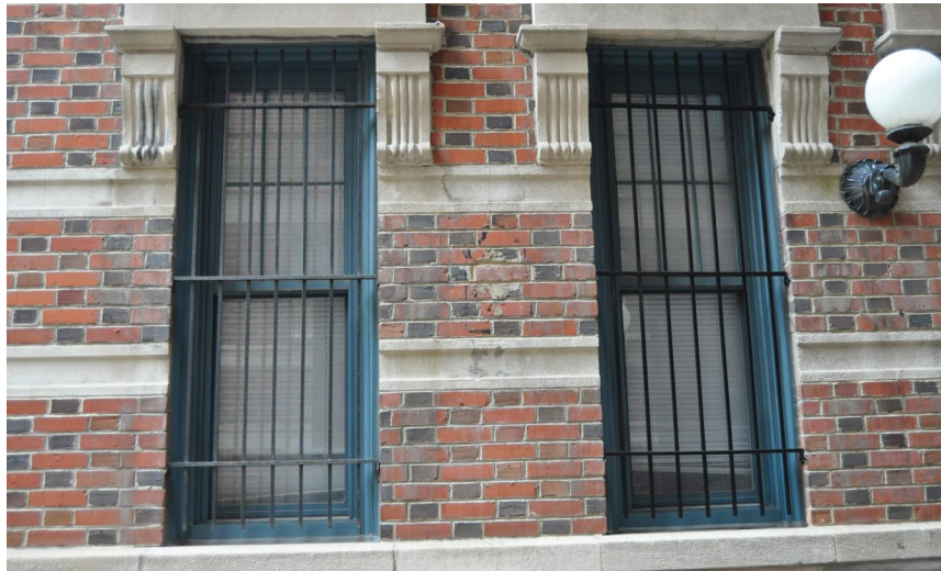
Security grilles attached at limited points to window surrounds at the ground floor.
