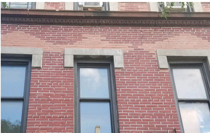
Example of a poor brick match. Note how the new bricks (above the lintels) do not match the historic bricks, calling undue attention to the repair.
