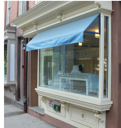
A fixed storefront awning installed at the top of the projecting display window.
