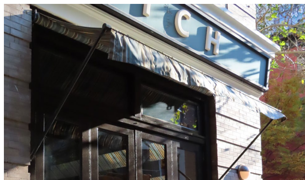
A retractable storefront awning installed at the top of the storefront infill within the opening.
