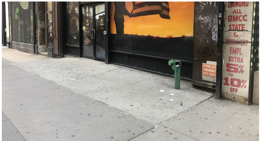
This concrete sidewalk has been sloped towards the storefront to make it accessible.
