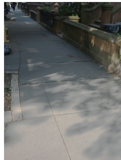
A new concrete sidewalk with saw-cut joints, tinted to match the adjacent historic bluestone.
