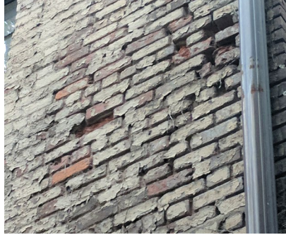
The coating used on the bricks resulted in severe deterioration of the brickwork.
