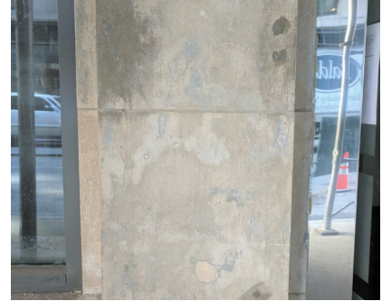
Coating would be appropriate in this case where cleaning revealed staining and previous repairs.
