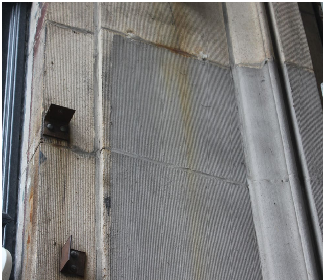
Example of inappropriate coating. In addition to being a poor color match, the coating extends over the mortar joints, sealing the masonry and mortar and restricting moisture transmission, which could accelerate deterioration.
