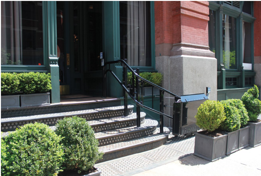
A chair lift on rails, finished to match the existing metal stairs and installed with minimal attachment points.
