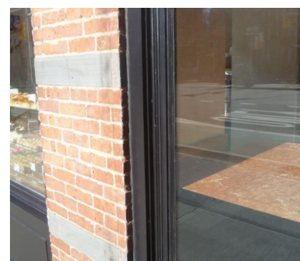
The molding profile used in this storefront recalls the articulation of historic storefront framing.
