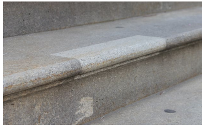
The light colored stone seen on the lower step is replacement stone installed as a Dutchman repair.
