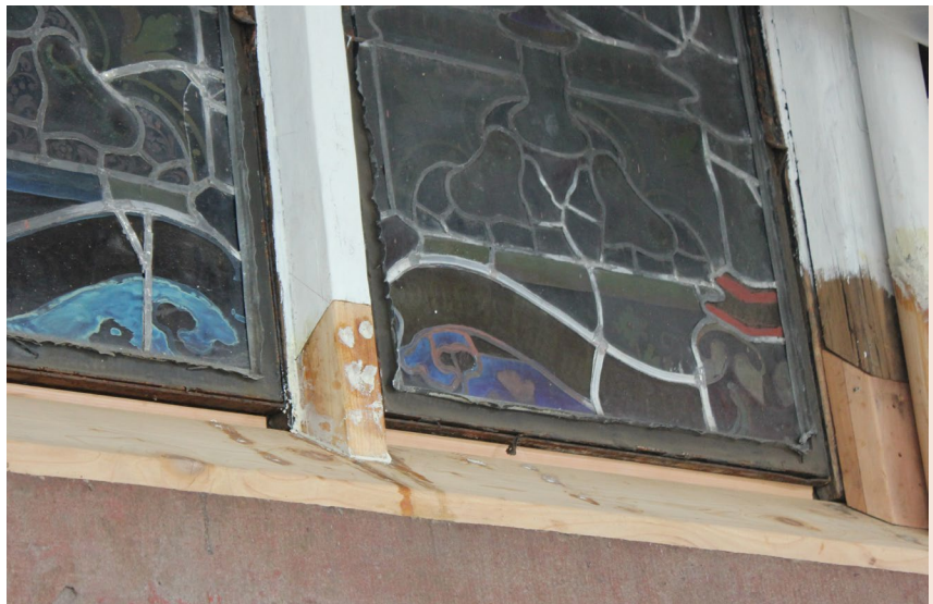
The wood mullions (vertical pieces of unpainted wood) have been repaired with a Dutchman repair. The new pieces of wood match the dimensions and profiles of the adjacent historic wood and will be repainted to blend in.
