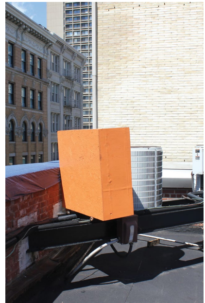
The orange box is a physical mock-up of a proposed rooftop HVAC unit. Staff may require such a mock-up to determine an installation's potential visibility from public thoroughfares.
