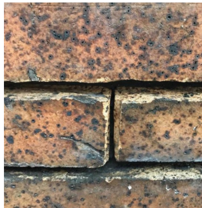
Inappropriate mortar joint removal. Note how the edges of the bricks have been damaged by the process.
