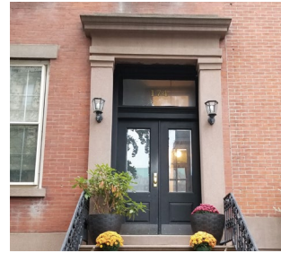
This replacement door recalls, but does not match, the historic door.
