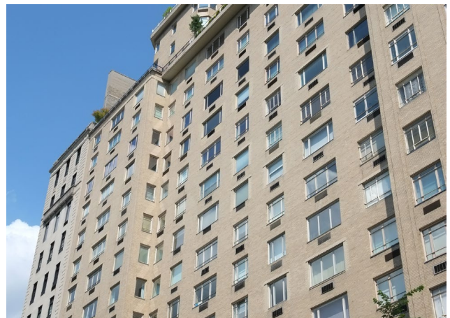
New installations should match an established regular pattern of through-wall HVAC installations.
