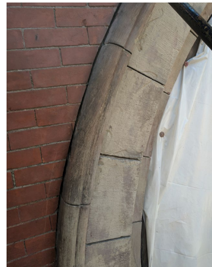
Historic masonry damaged by harsh coating removal and cleaning methods
