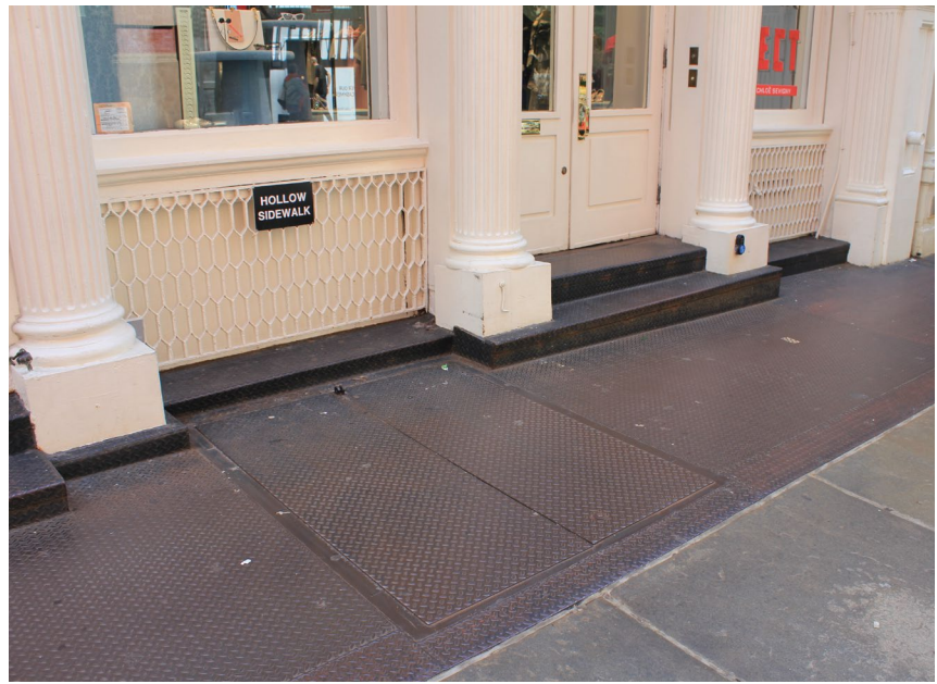
Deteriorated historic vault lights can be covered and protected by steel diamond plate with a dark painted finish, as seen here.
