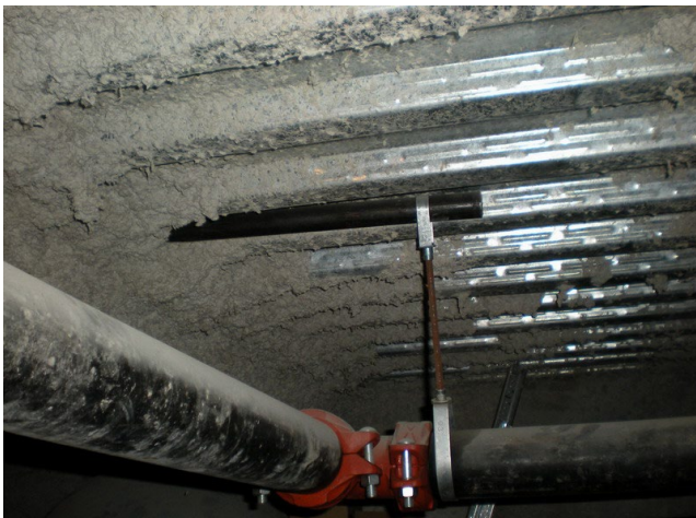
Sprinkler System Improper Hanger
