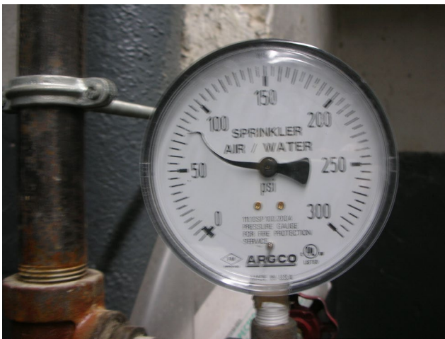
Defective Water Pressure Gauge
