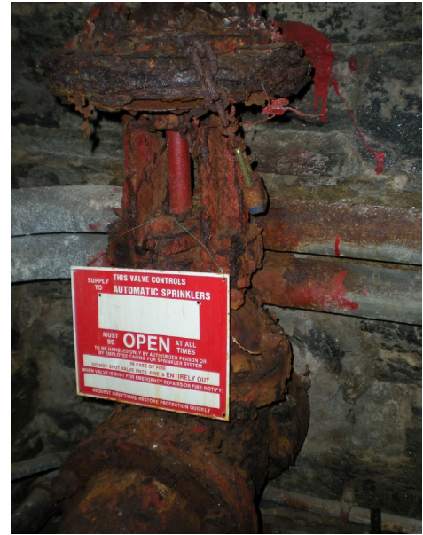
Corroded Curb Valve in Sidewalk Vault
