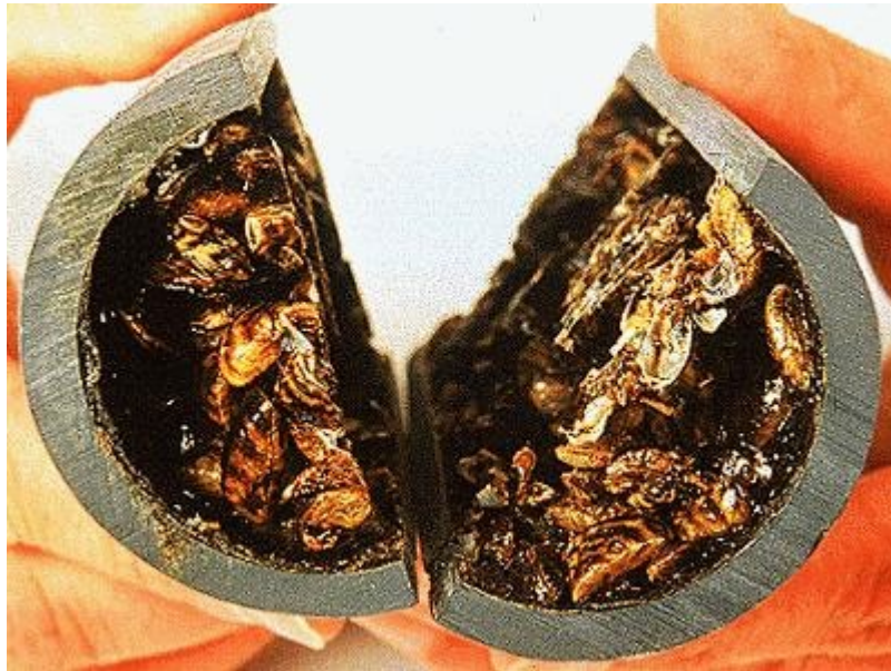
Piping Infested with Zebra Mussels
