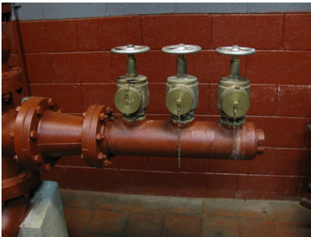
Fire Department Test Manifold
