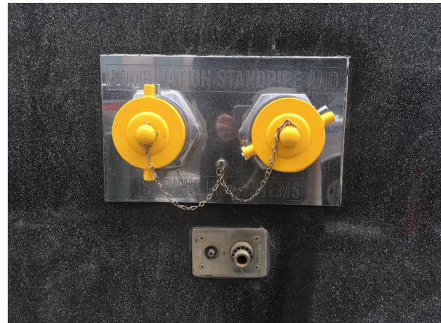
Sprinkler & Standpipe Fire Department Connections
