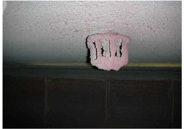
Loaded Sprinkler in Head Cage Head
