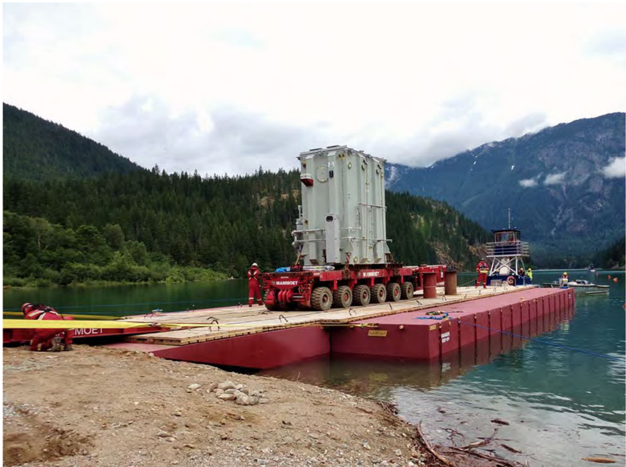
Figure #4 Representative FlexiFloat Units Configured as a Floating Construction Dock
