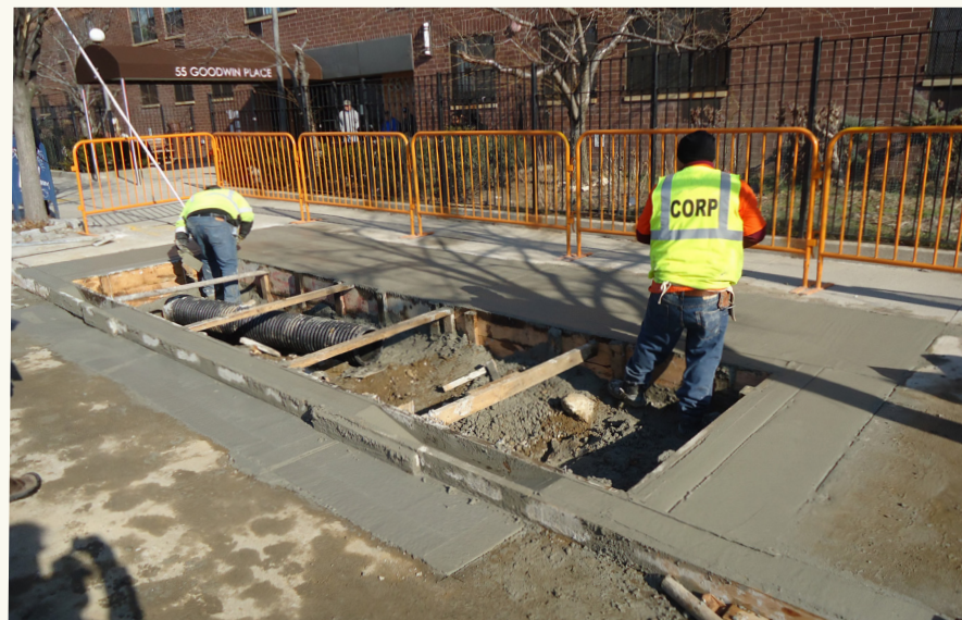
CONTRACTORS FINISH A CONCRETE EDGE AND REPLACE THE SIDEWALK AROUND A NEW RAIN GARDEN
