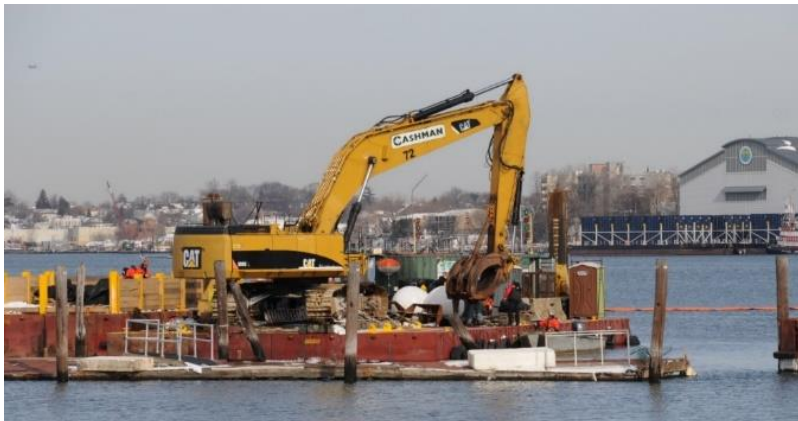
Environmental Dredging: Proposed location head of Bergen Basin but final locations TBD
