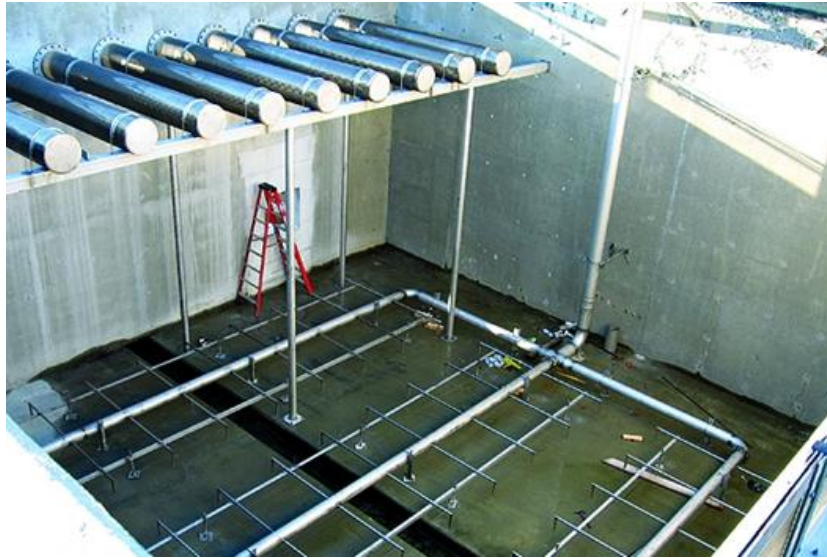
Figure 3-8: IFAS Installation with Growth Media (Gellner 2014)
