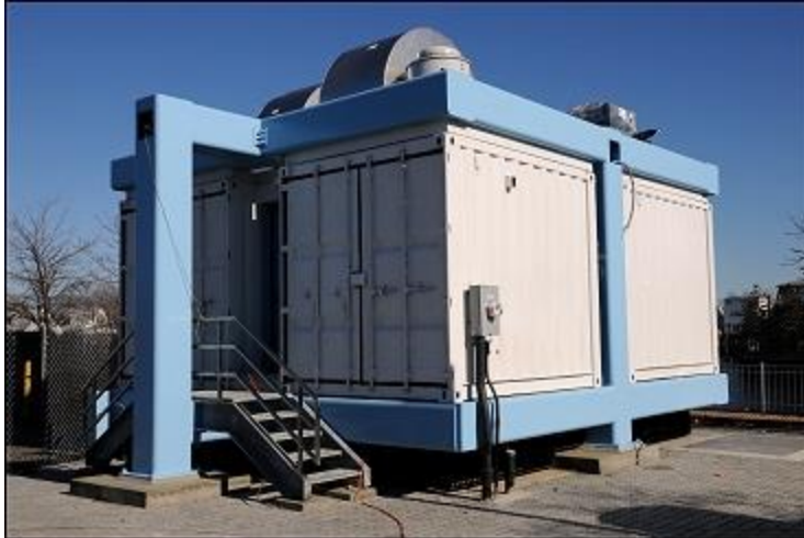
Figure 6-14: Shellbank Basin Destratification Facility
