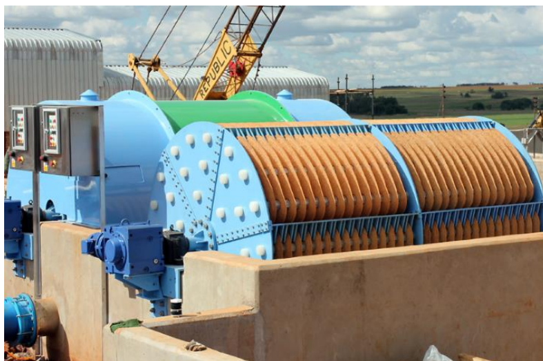
Figure 3-7: HYBACS RBC System (Bluewater 2011)
