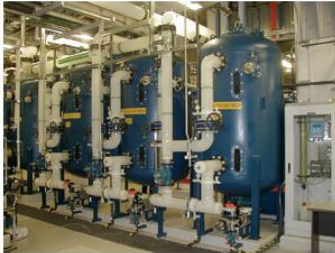
Figure 3-9: Ion Exchange Vessels (Gunderson 2014)
