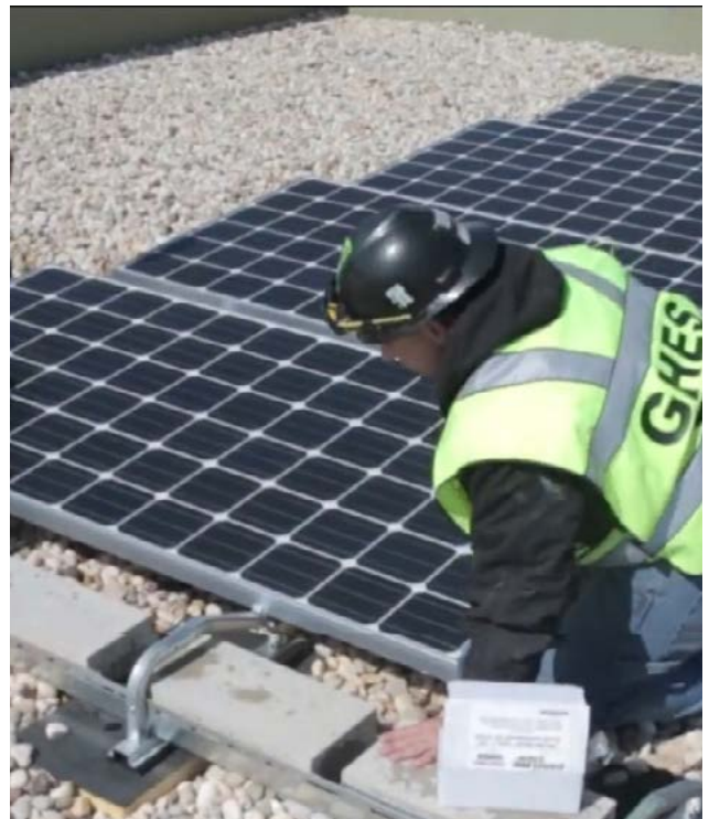
Solar installation in NYC
