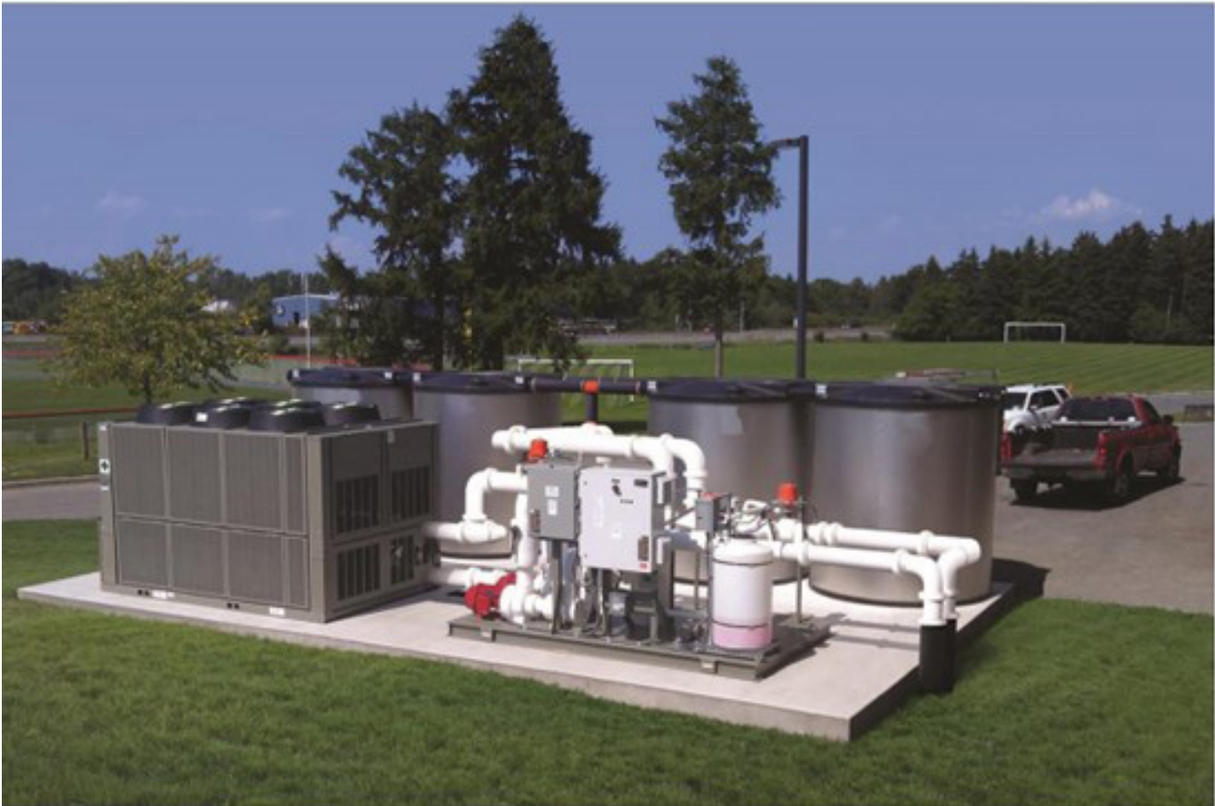
Figure 8: Trane® Thermal Energy Storage, Jefferson Community College, Watertown, NY 19
