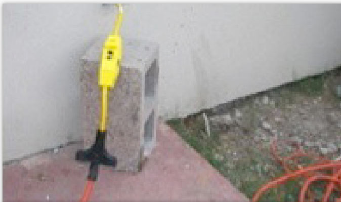
Protect extension cords at the power source by using a Ground Fault Circuit Interrupter (GFCI)
