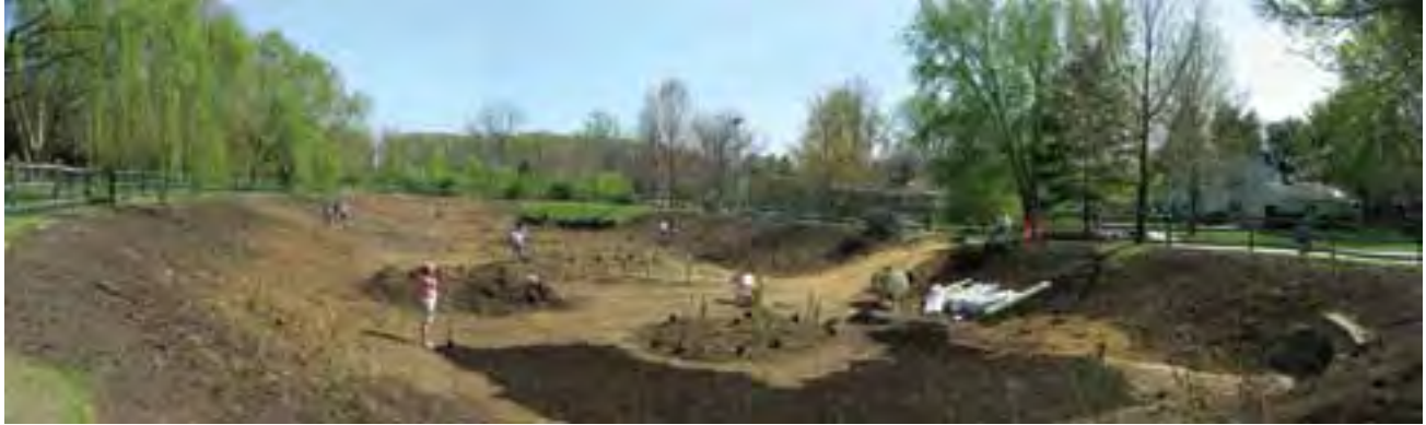
Leaf litter from local residents was added to enrich soils at this stormwater detention basin, helping a diverse range of newly planted vegetation to thrive.
