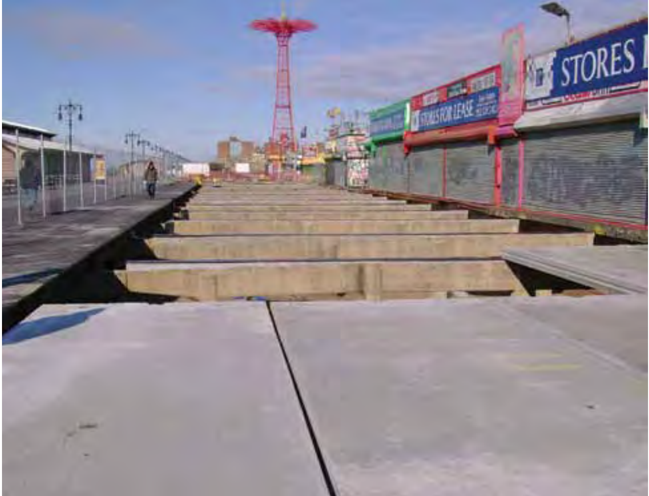
The Parks Department used recycled fly ash, an industrial byproduct, in new concrete boardwalks throughout New York City, including this one at Coney Island.
