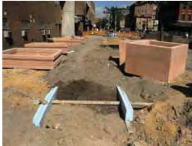
Existing urban soils at the project site were amended to improve soil quality while minimizing importation of new soils.
