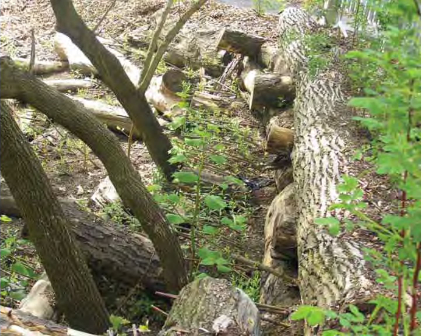
At Pugsley Creek Park in the Bronx, retaining walls incorporate willow braches that will continue to grow, providing greater soil stabilization and habitat.
