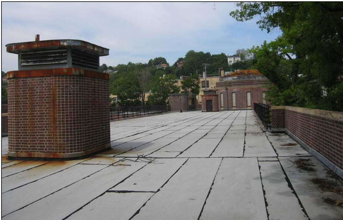
Tompkinsville (Joseph H. Lyons) Pool: Roof deck showing fan rooms and rotunda clerestory and dome roof (view looking west) Photo: Tara Harrison, 2008
