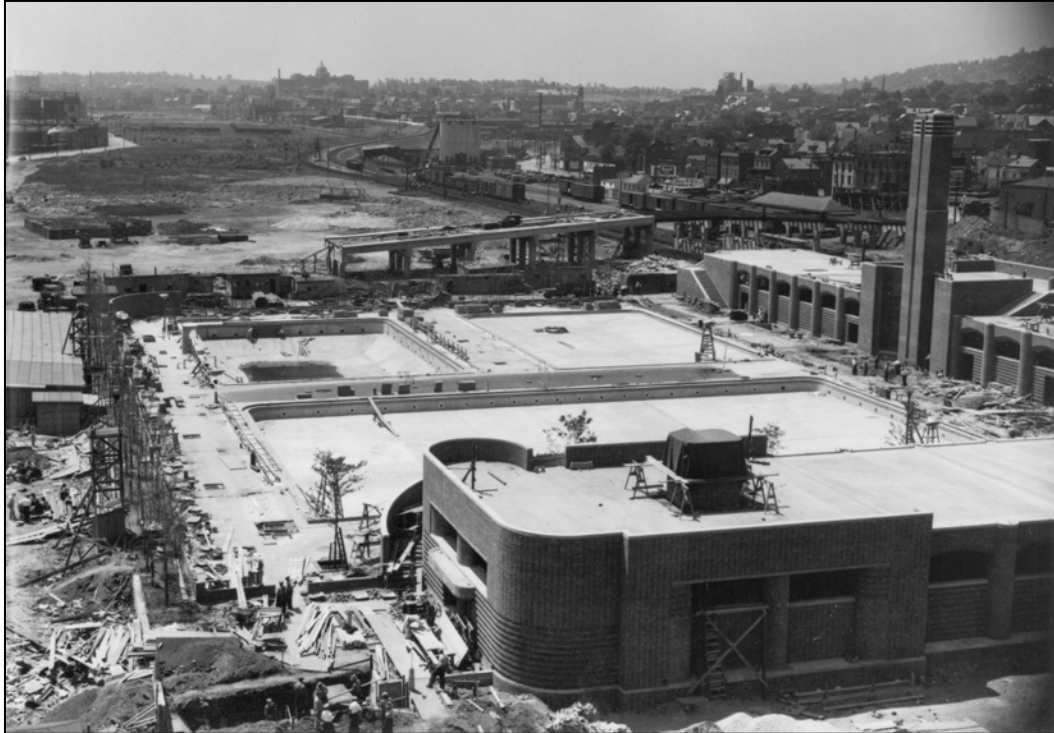
Tompkinsville (Joseph H. Lyons) Pool during construction 1936 (view looking south) Photo: New York City Parks Photo Archive
