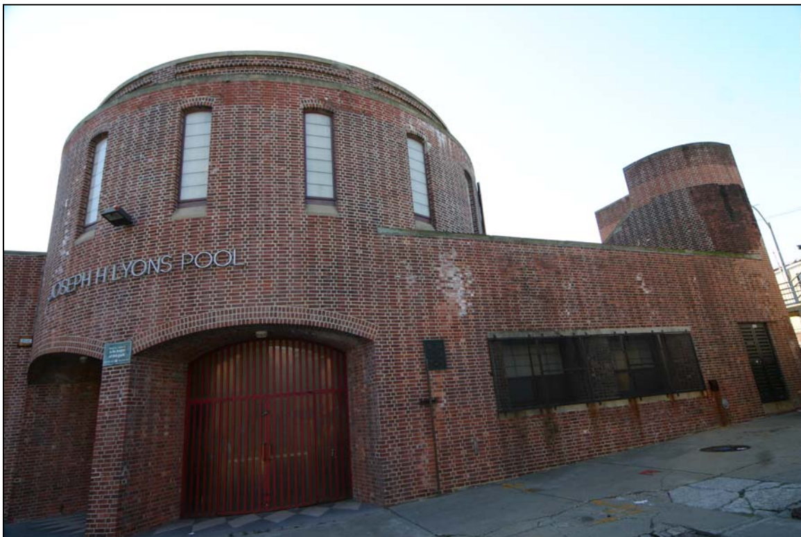
Tompkinsville (Joseph H. Lyons) Pool: Rotunda and westernmost portion of north facade Photo: Carl Forster, 2007
