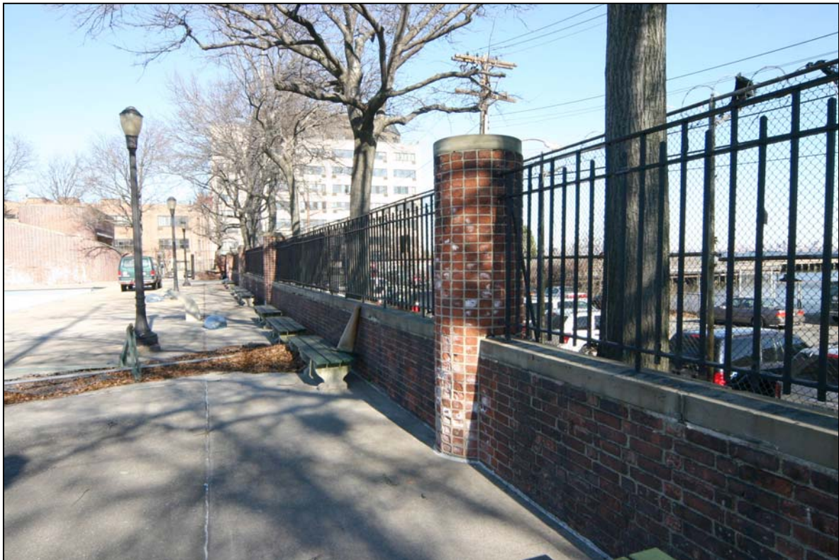
Tompkinsville (Joseph H. Lyons) Pool: Pool deck fencing (view looking north) Photo: Carl Forster, 2007
