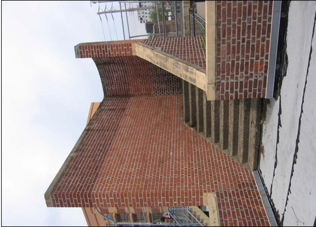
Tompkinsville (Joseph H. Lyons) Pool: Roof stair to footbridge Photo: Tara Harrison, 2008
