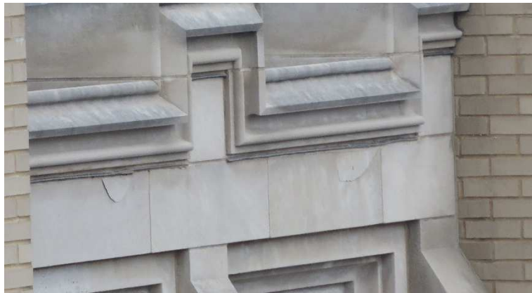
Masonry cracks and spalls
