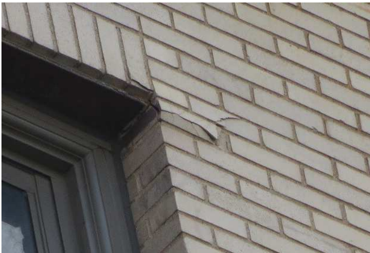
Brick bulging and open joints Corroding steel lintel
