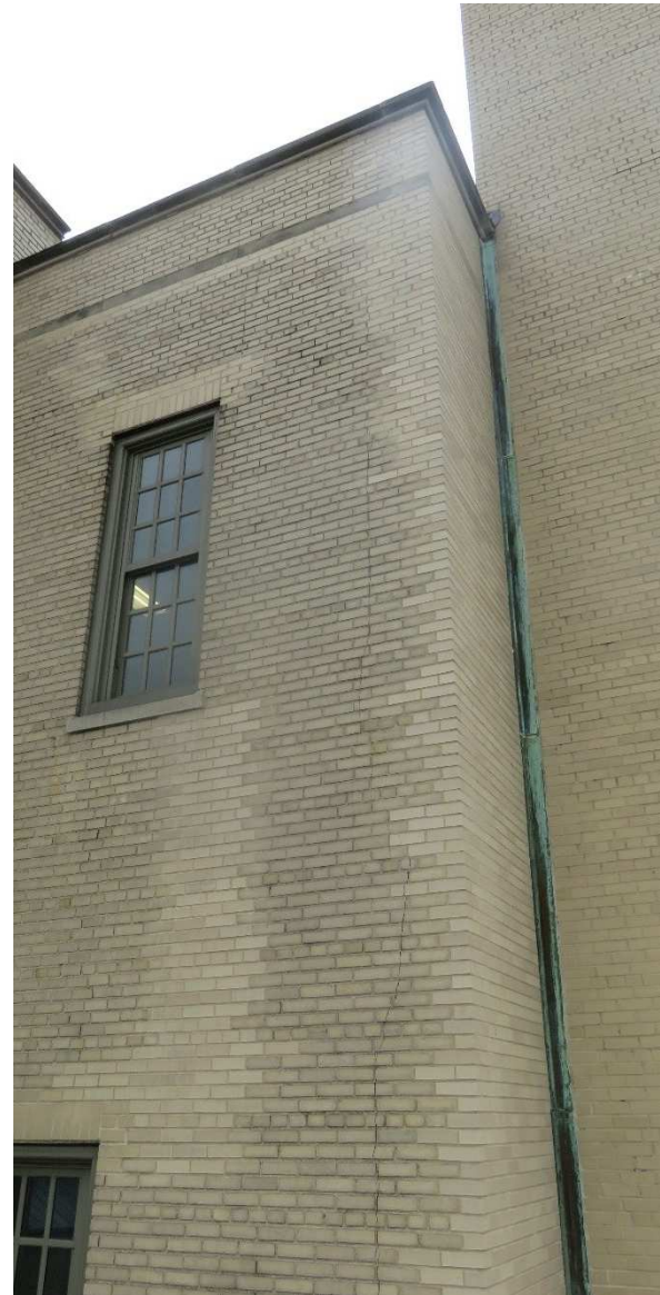
Large vertical crack at corner
