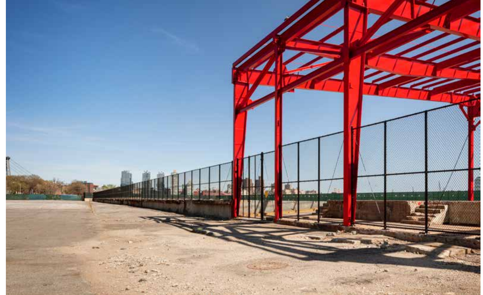
2 View east showing full expanse of deck. Western deck access is visible beneath the shed structure.
