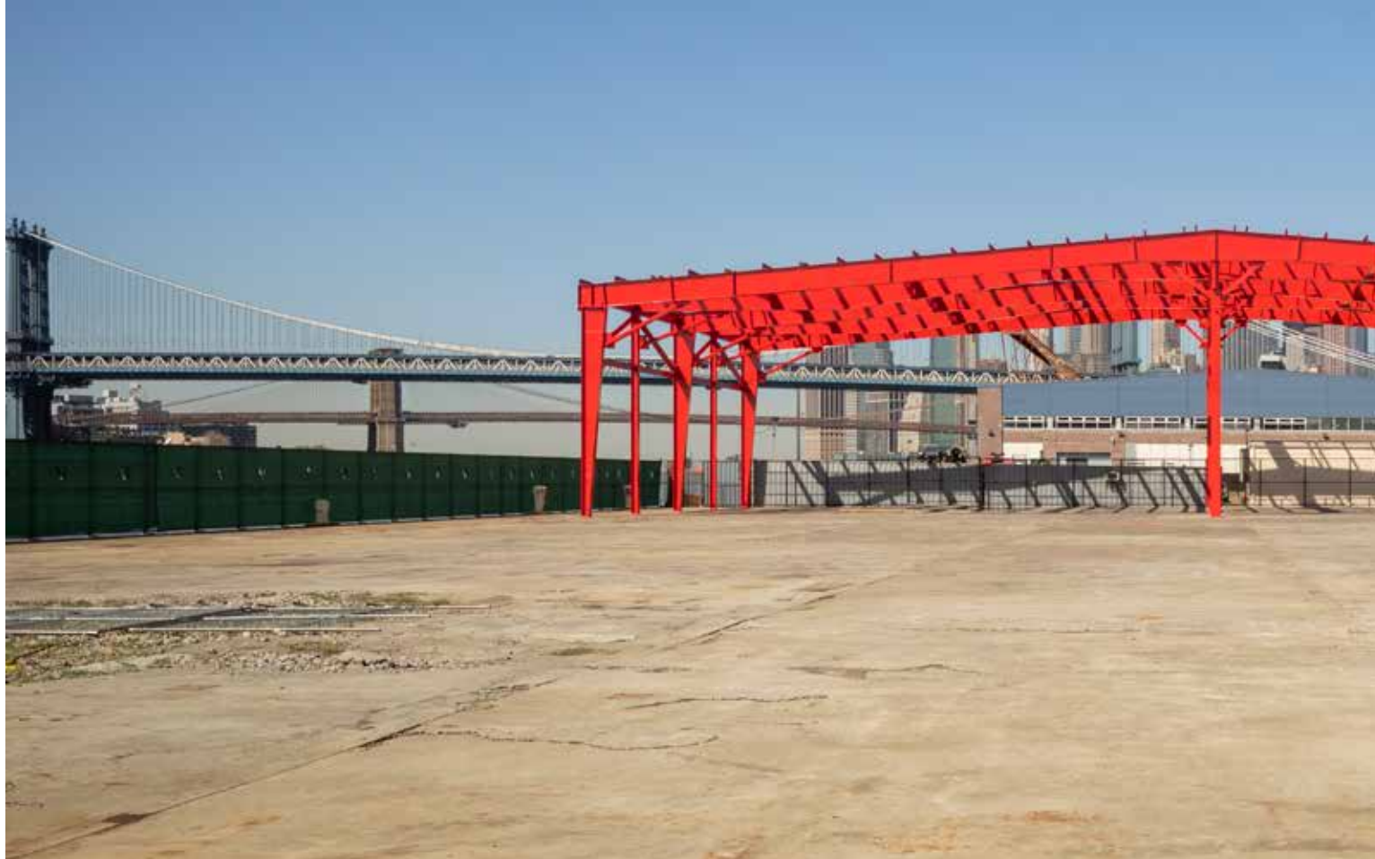
1 View west towards the existing shed frame (painted red). Spalling concrete condition is visible in the foreground and the existing boat cleats are visible along the fenceline.
