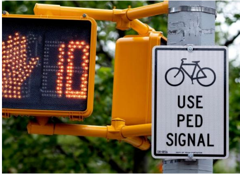
Traffic Control Signals & Timing
