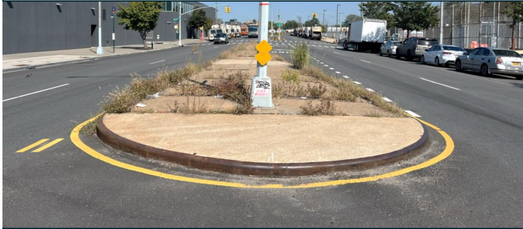
The existing medians are substandard
