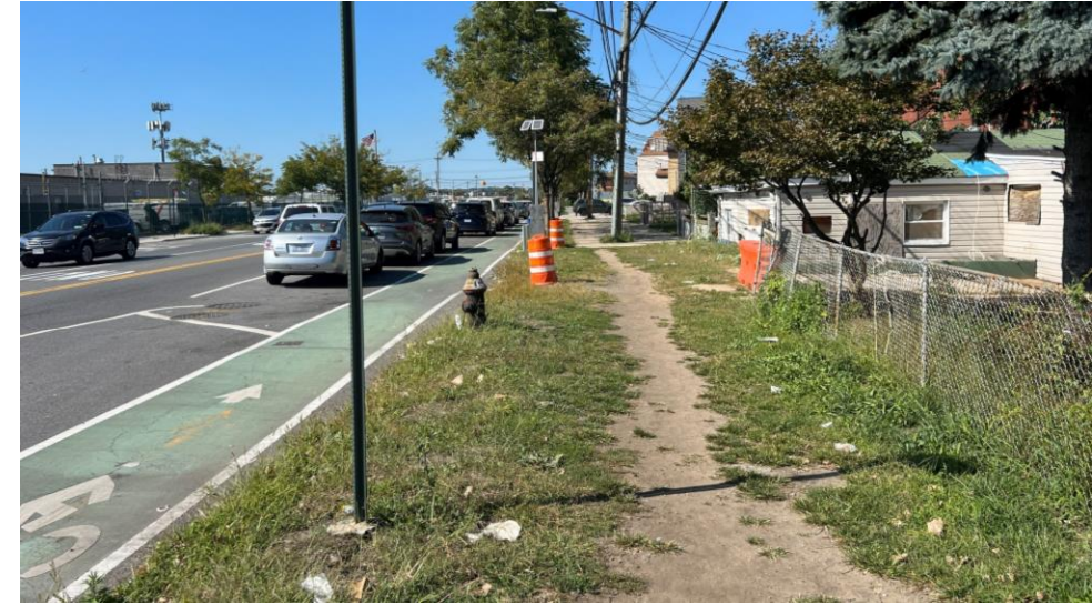
Concrete sidewalk missing at Fountain Ave
