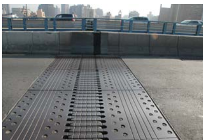
Manhattan Bridge Finger Dam. (Credit: Jagtar Khinda)
