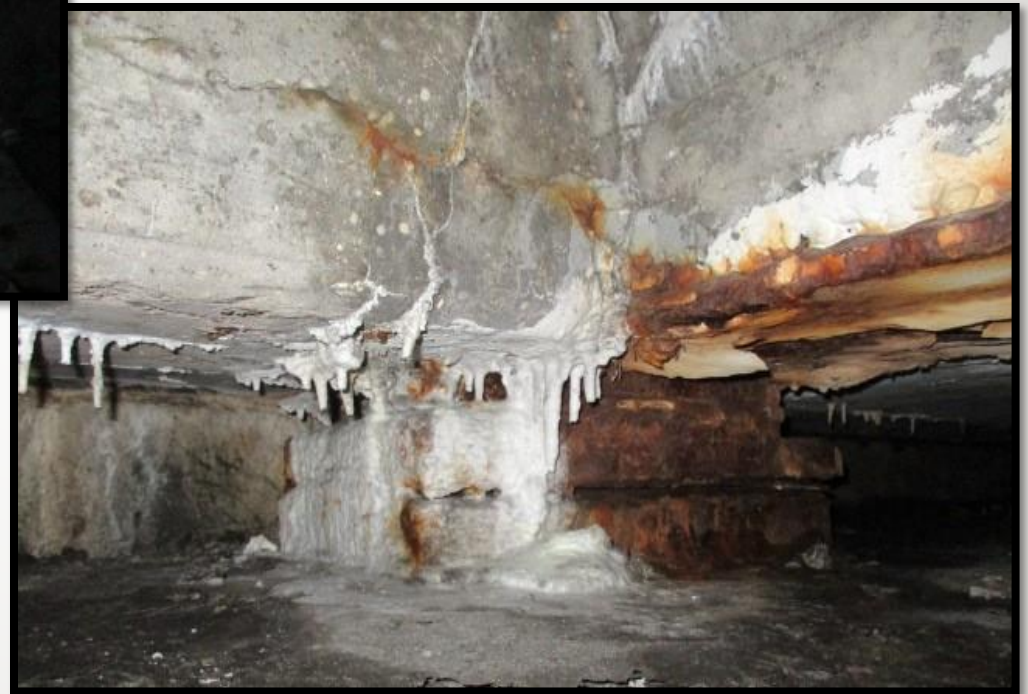
Deteriorated Steel Rocker Type Bearing
