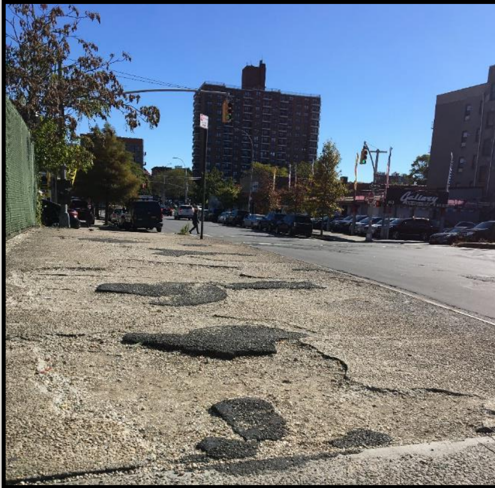
Pot holes and patching in sidewalk
