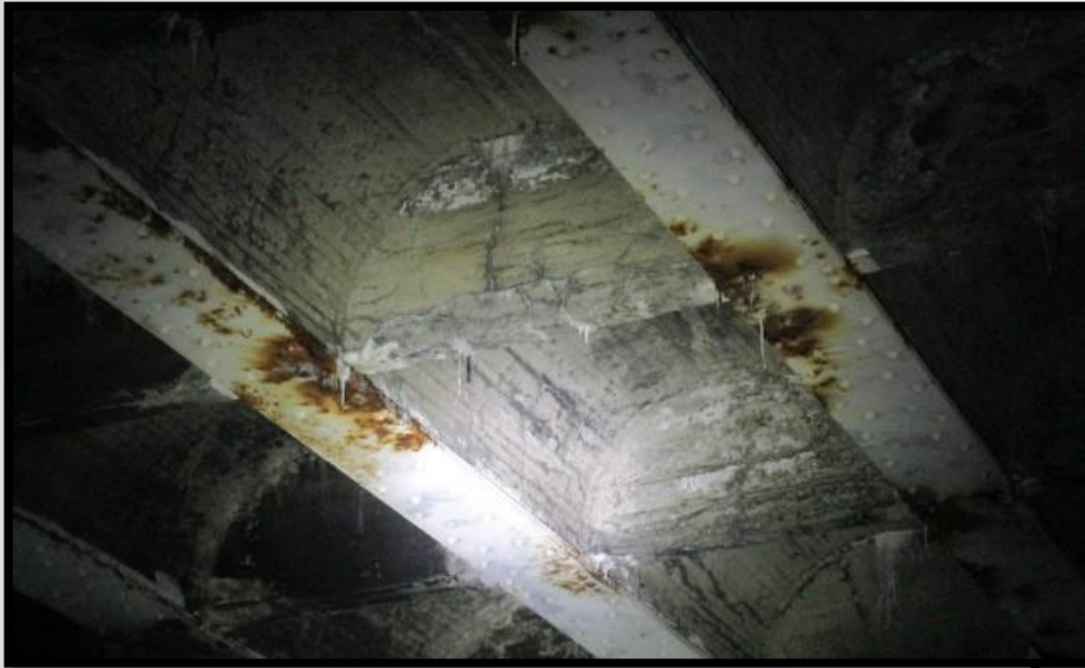
Deteriorated Underside of Deck Corrosion of bottom flange of steel girders, cracking of structural deck and concrete encasements.
