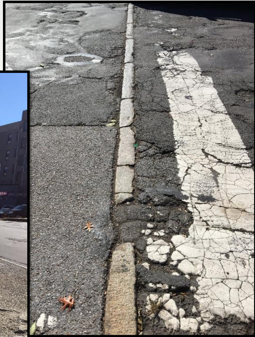
Deteriorated joints, map cracking & settlement
