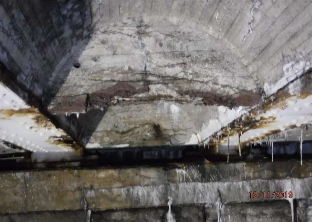
DETERIORATED CONCRETE BELOW DECK (DEBRIS FALL ON MNRR TRAINS)
