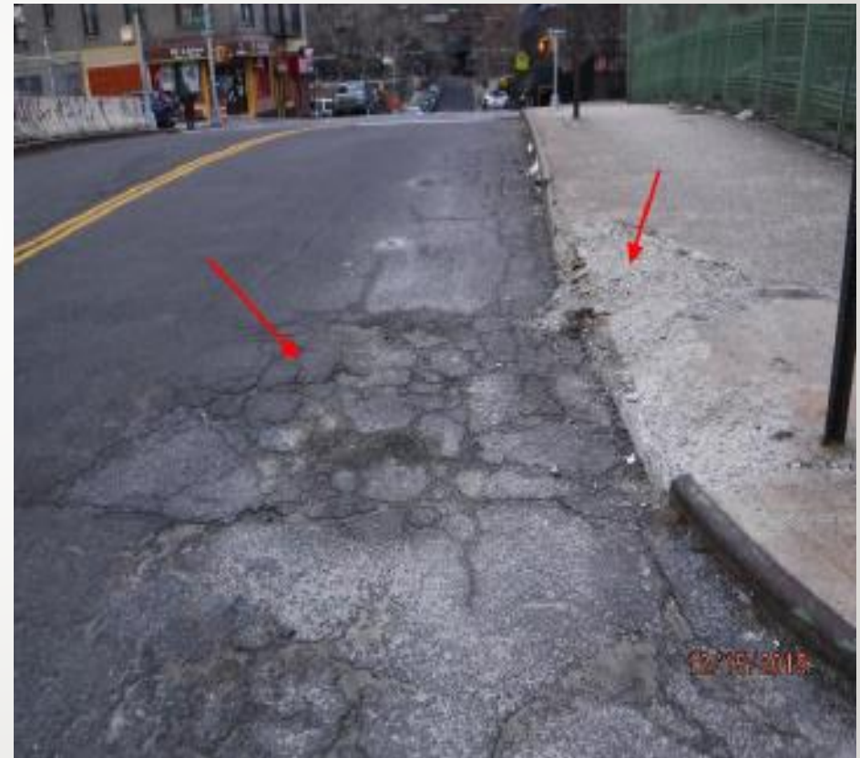
DETERIORATED PAVEMENT SPALLED SIDEWALKS
