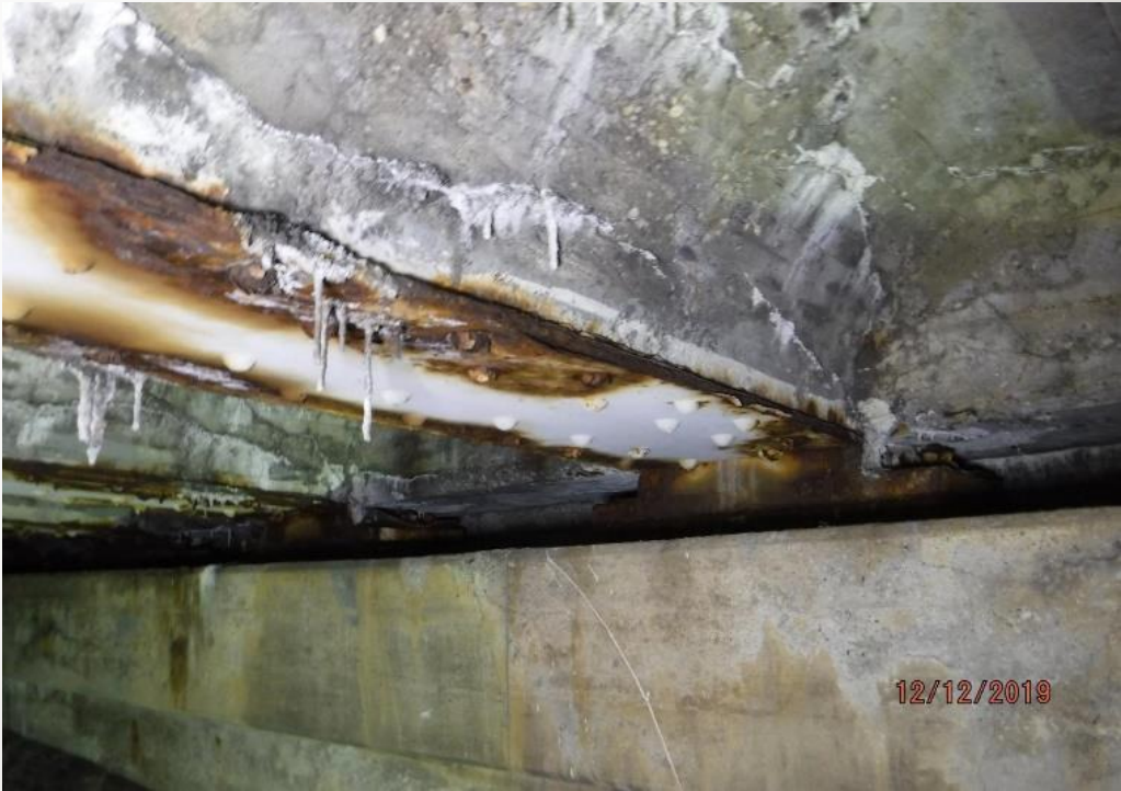
CORROSION AT GIRDER (VISIBLE BOTTOM FLANGE)
