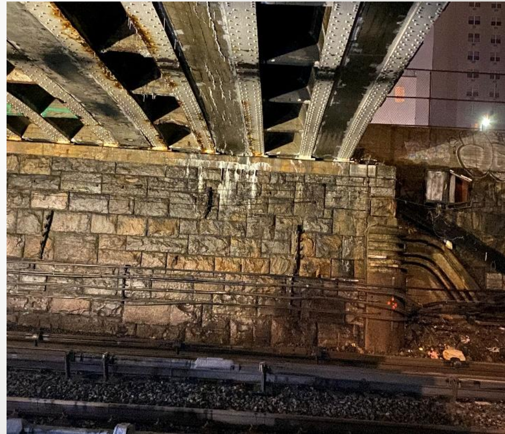
ABUTMENT STONE JOINTS IN POOR CONDITION
