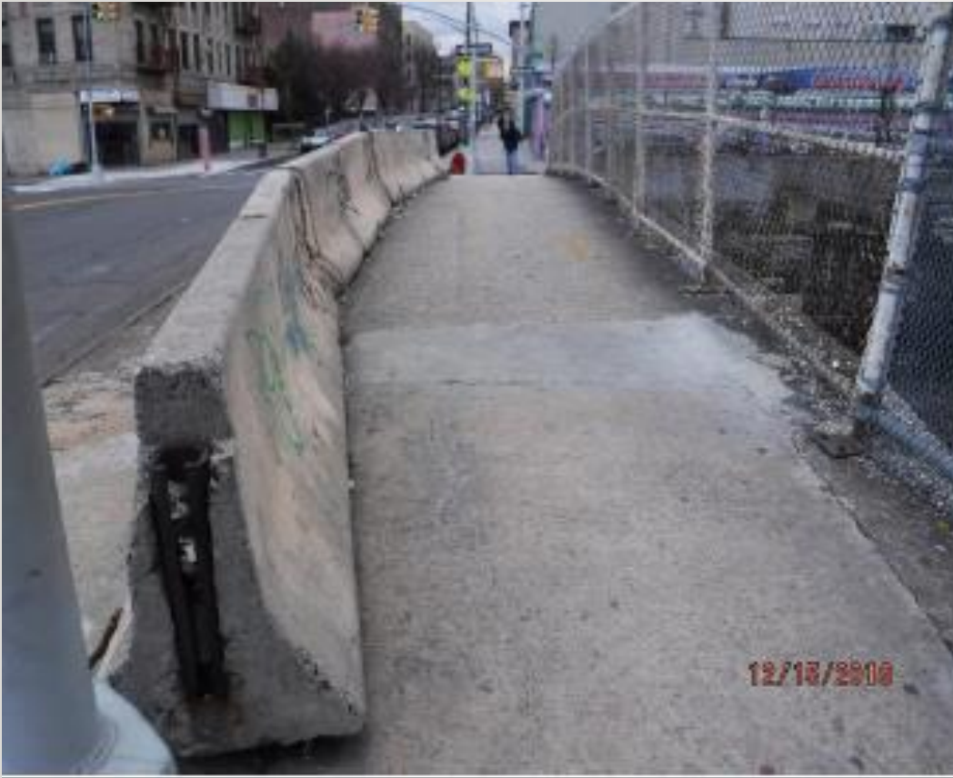
NO TRAFFIC RAILING AT SOUTH SIDEWALK
