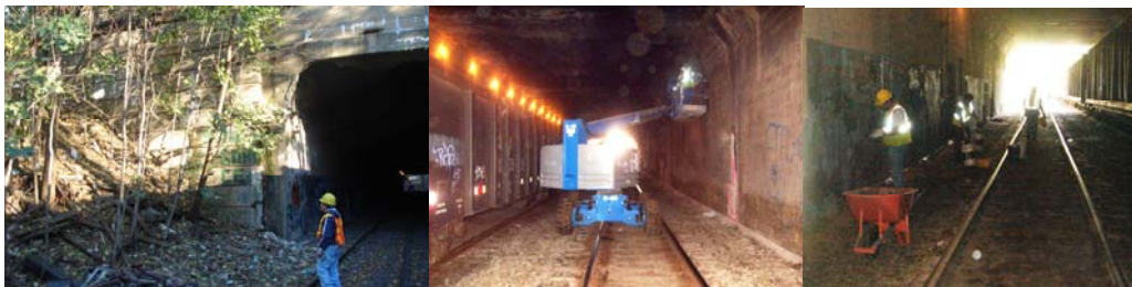
Inspecting Conditions at the Metropolitan Avenue Bridge in November 2006. Working Under the bridge in December 2006. Underdeck Repair Work in June 2007.
