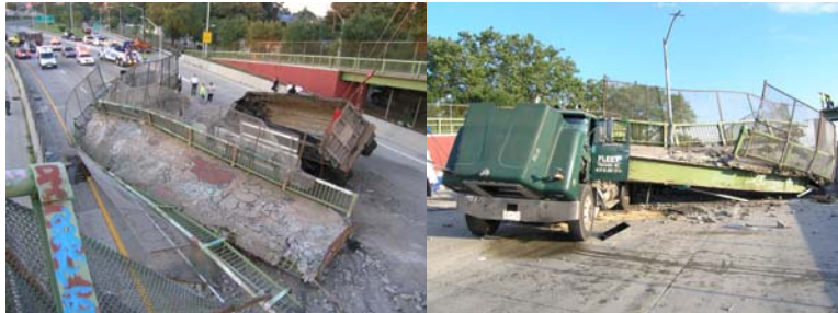
Waterbury Avenue Bridge Damage.
