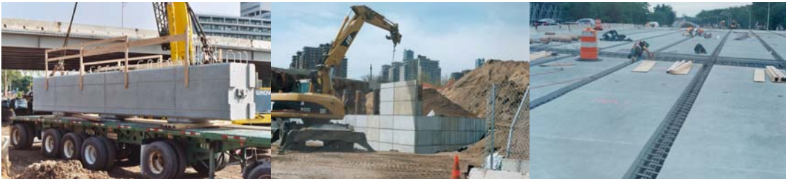
Precast Pier Capbeam Section Prior to Setting it on the Cast-in-Place Columns. Installing T-Walls. Precast Panels and Joints Awaiting Cast-in-Place Concrete Placement.
