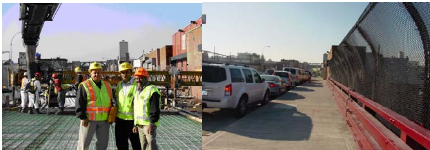
Project Engineer Ashraf Anis, Director of Component Rehabilitation Krishan Baweja, and Project Manager Rezaul Karim at the site in April 2008. North Sidewalk Looking West After Rehabilitation.
