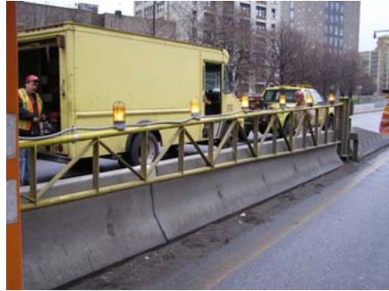
Electricians Thomas Cipriano and Robert Stackpole Inspecting the Repaired Lights. (Credit: Hany Soliman)
