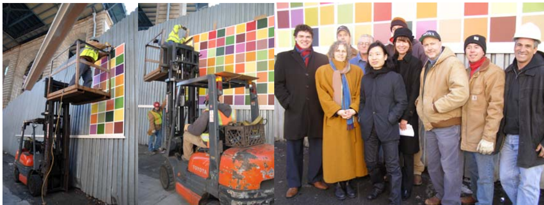
Installing the Mural Panels on February 21, 2008. Celebrating the Installation of the Temporary Art Program Mural in DUMBO are, From Left to Right: DUMBO Improvement District Executive Director Tucker Reed, Supervisor Bridge Repairer and Riveter John Jones, Assistant Commissioner of Urban Design and Art Wendy Feuer, Bridge Repairer and Riveter David Collins, Mural Artist Tattfoo Tan, Carpenter Joseph Moschella, Commissioner Janette Sadik-Khan, Carpenter Stephen Buckley, Carpenter William Sic, and Supervisor Carpenter Joseph Vaccarro.
