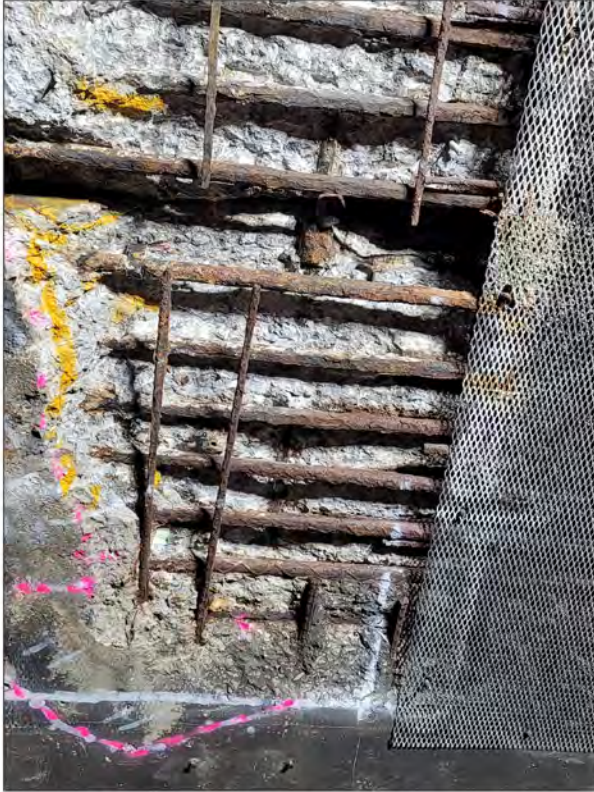
1 Reinforced concrete deck soffit showing spalled concrete, exposed, and corroded concrete reinforcement bars, efflorescence, and scaling. This condition is typical at underside of deck relief joints. Photo taken during recent interim repairs with removal of unsound concrete in progress.
