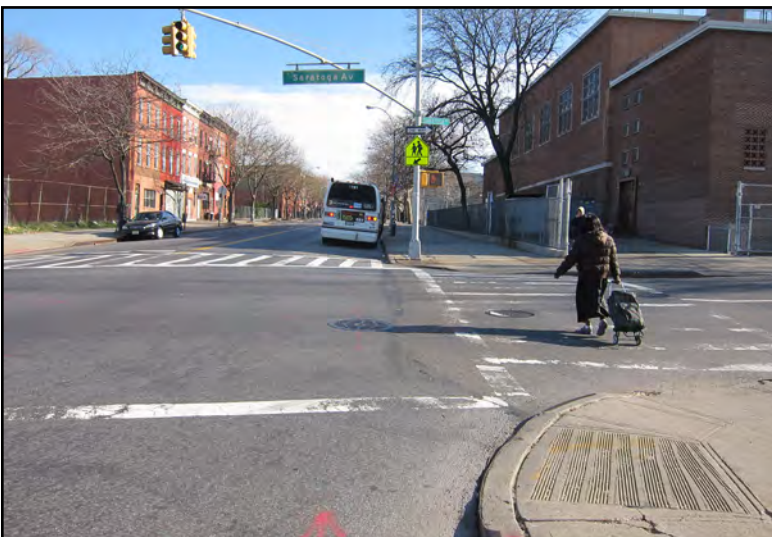
Before: Faded markings at intersection
