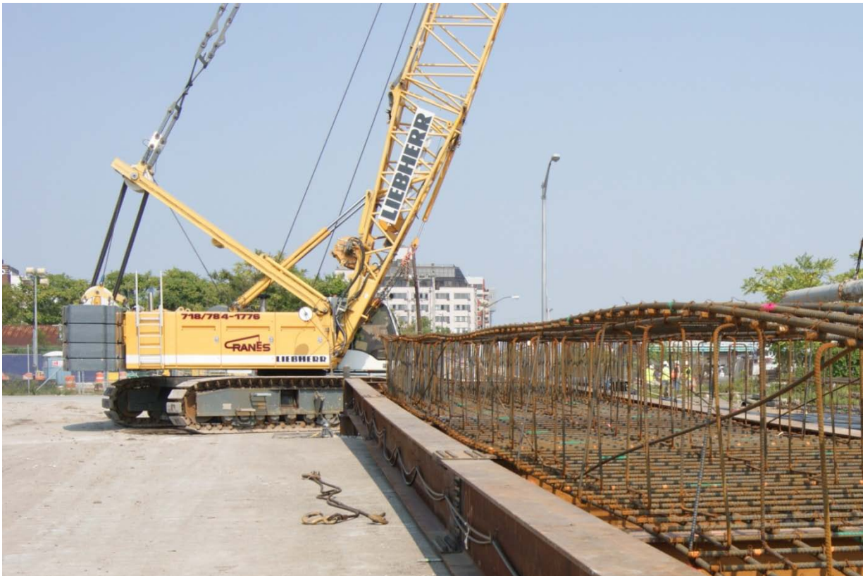
Slurry wall panel on lifting frame prior to transport across Front Street to shaft site
