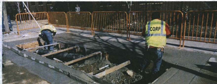
CONTRACTORS FINISH A CONCRETE EDGE AND REPLACE THE SIDEWALK AROUND A NEW RAIN GARDEN
